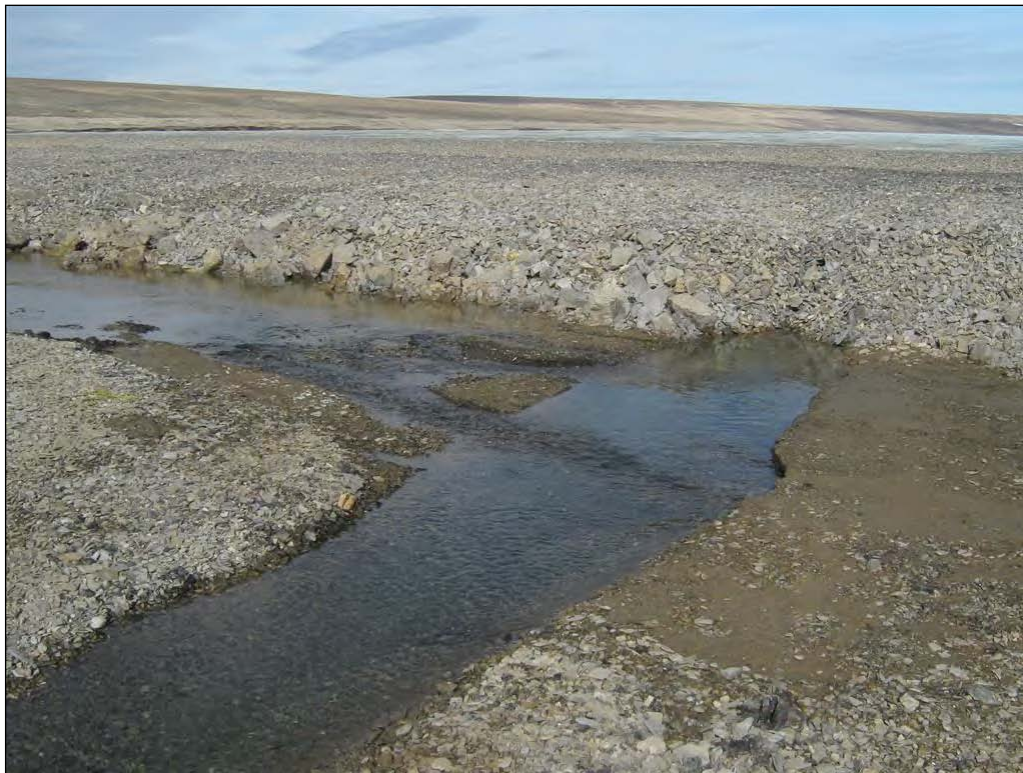
Photograph 23. Wave Break Structure, seepage through rockfill at east end of former wave break ↑
