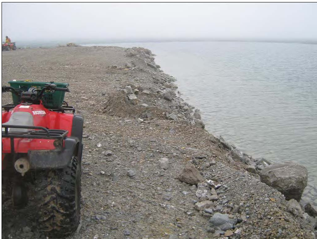
Photograph 70. Frustration Lake Jetty, shifted rockfill from ice action on East side of jetty ↑
