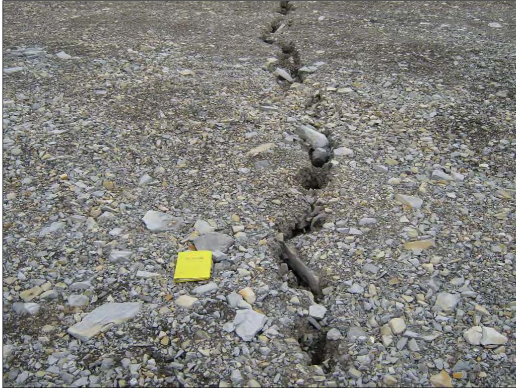
Photograph 29. Subsidence Area, previously observed tension crack (no change) ↑
