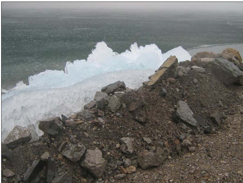
Photograph 72. Frustration Lake Jetty, shifted rockfill from ice action at North end of jetty ↑
