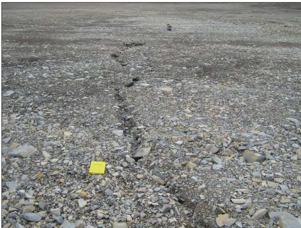
Photograph 28. Subsidence Area, previously observed tension crack (unchanged) ↑
