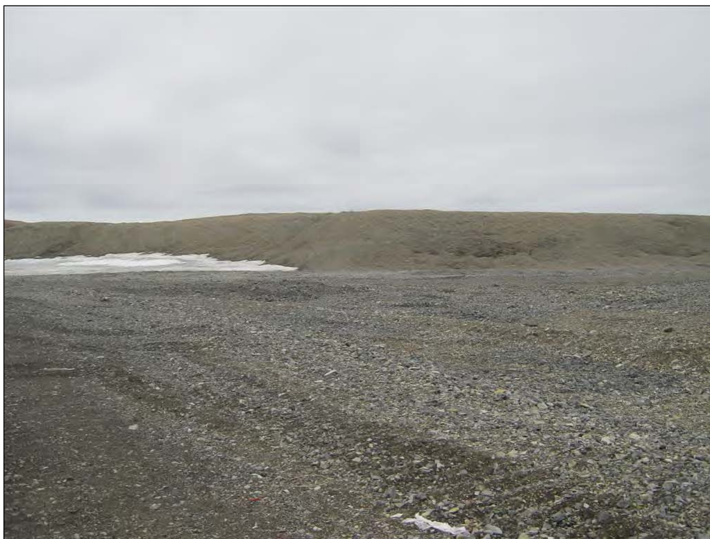
Photograph 57. New Quarry, West perimeter slope with minor settlement on lower half of slope ↑
