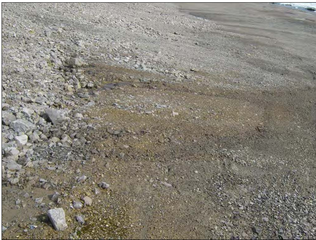
Photograph 14. Operational Landfill, Seepage from SE toe ↑
