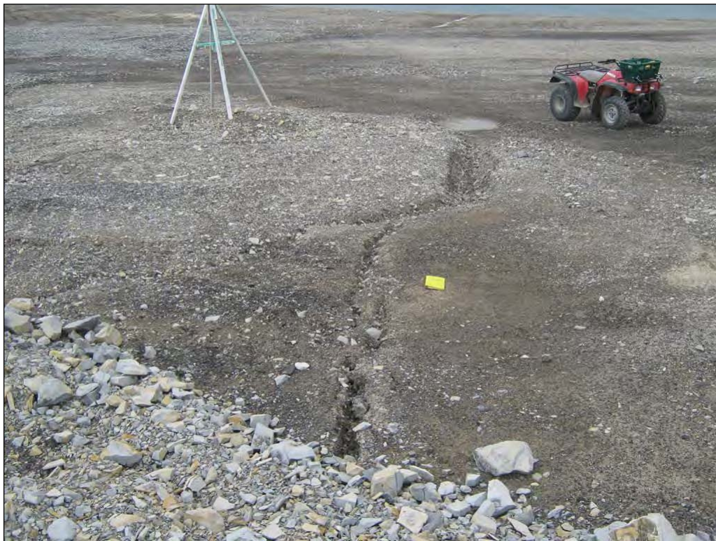
Photograph 30. Subsidence Area, previously observed tension crack (no change) ↑
