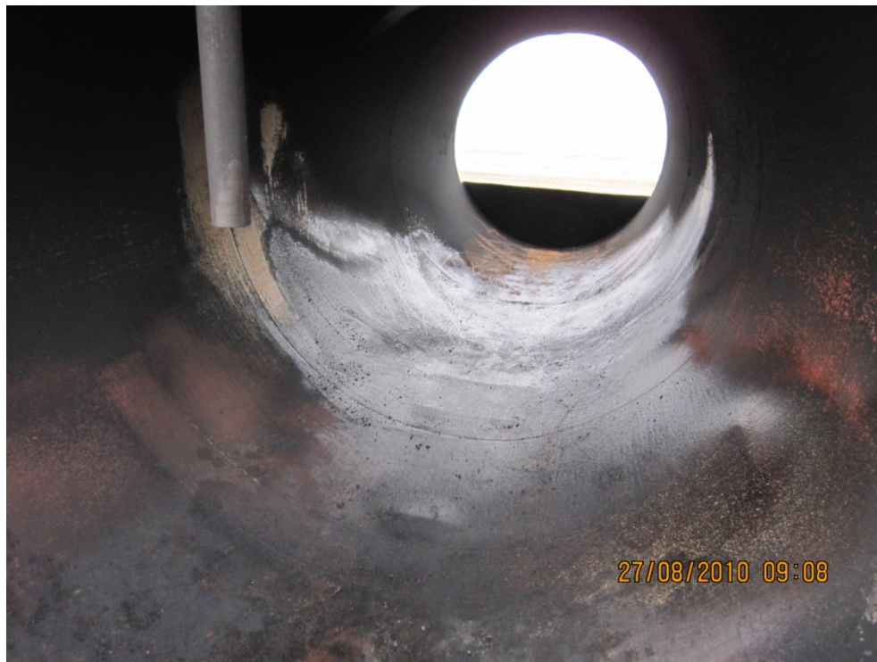
Photo #33 – Fuel Tank After Being Wiped Clean
