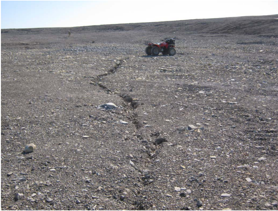
Photo 57, Subsidence Area, Central backfilled area, Old tension crack (~30m x 0.3m)
