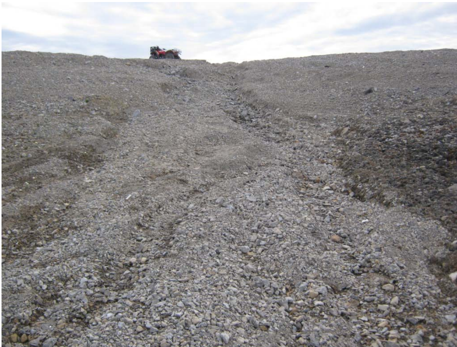
Photo 117, Frustration Lake, Self-armouring erosion gully on west side of road
