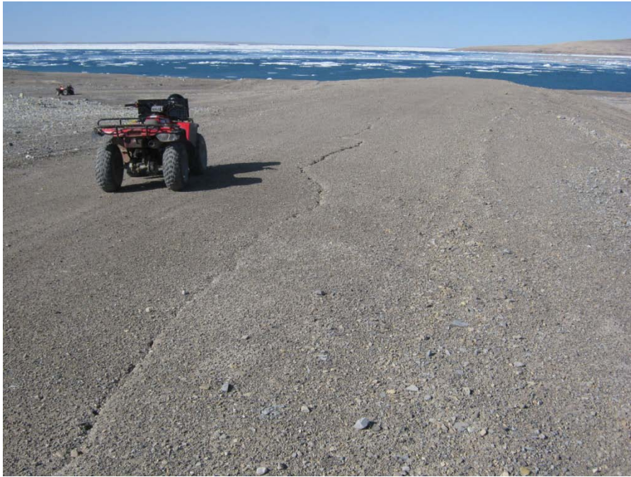
Photo 61, Subsidence Area, Tension crack on road west of New Quarry (~25m x 0.1m)
