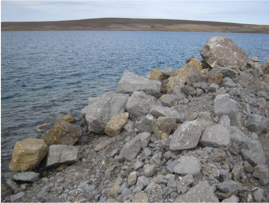
Photo 121, Frustration Lake, North end of the jetty (rockfill pushed by ice)
