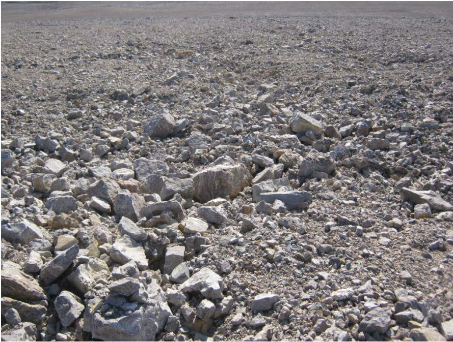
Photo 5, Operational Landfill, Central Slope, Undulations (~0.5 m deep) at top of slope
