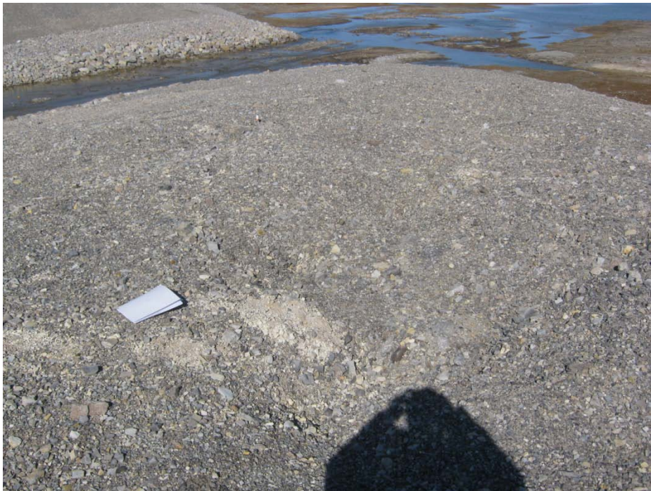
Photo 34, Garrow Lake Dam, East abutment crest, Minor settlement (8.5"x11" book for scale)
