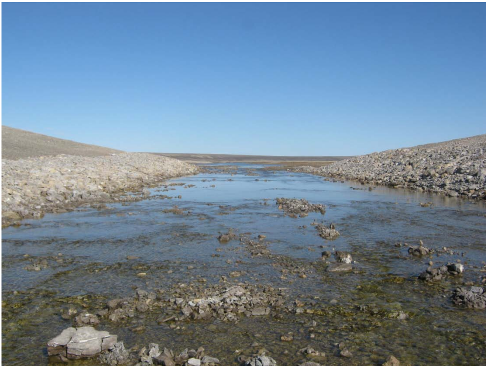
Photos 30, Garrow Lake Dam, Creek, Facing upstream through breach
