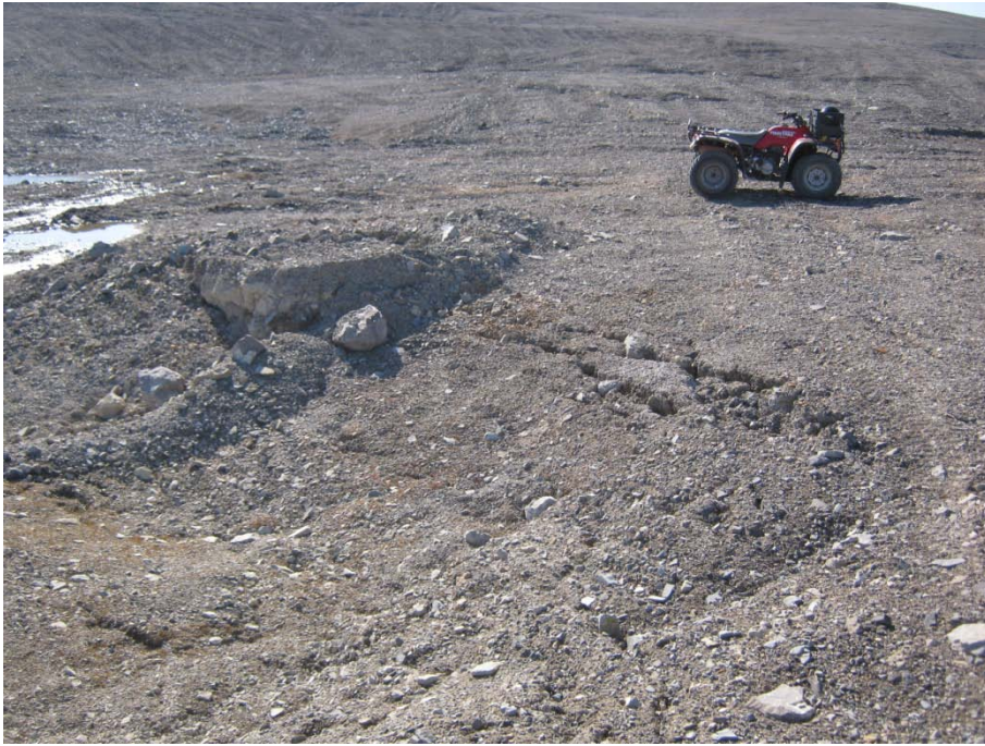
Photo 63, Subsidence Area, North of ponded water, Thaw settlement (~10m x 5m x 1m deep) beside backfilled vent raise
