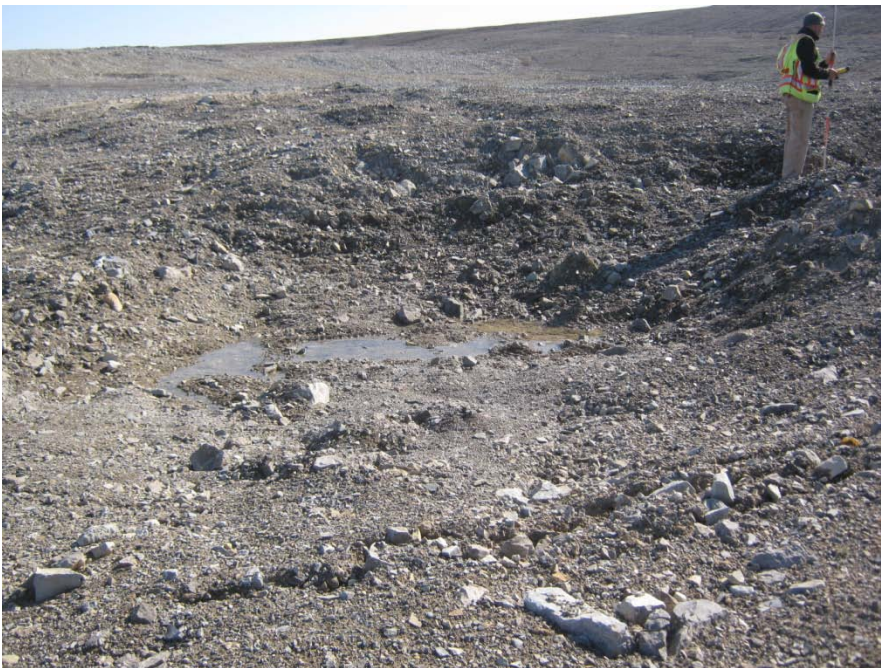
Photo 66, Subsidence Area, Northeast end, Thaw settlement (~10m x 10m x 1m deep)
