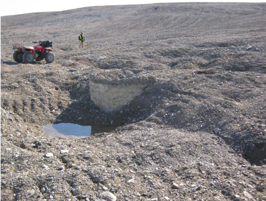
Photo 65, Subsidence Area, West of ponded water, Thaw settlement (~5m x 5m x 1m deep) beside backfilled vent raise
