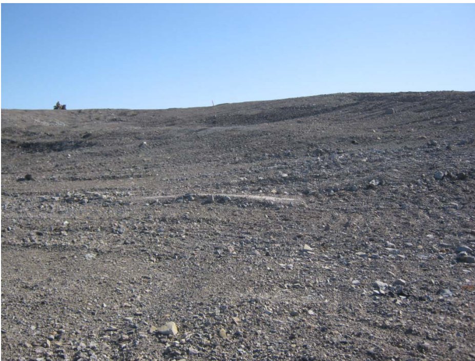
Photo 52, Subsidence Area, Northwest end, Facing South
