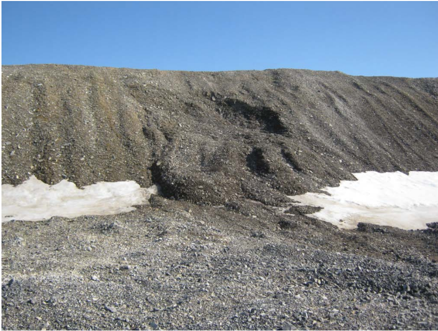
Photo 75, New Quarry, South perimeter slope, Minor slumping and erosion of slope bottom
