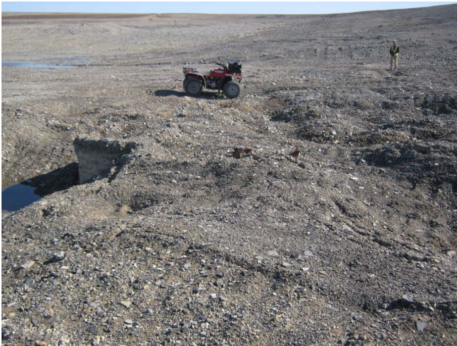
Photo 64, Subsidence Area, West of ponded water, Thaw settlement (~5m x 5m x 1m deep) beside backfilled vent raise
