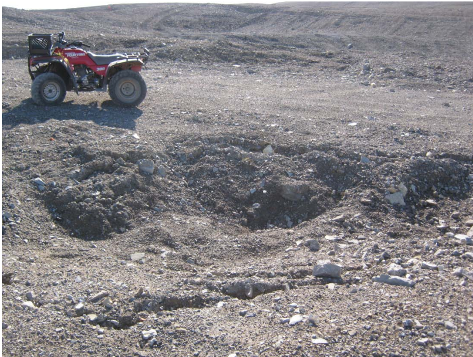
Photo 54, Subsidence Area, North end, Thaw settlement (~8m x 5m x 1m deep)
