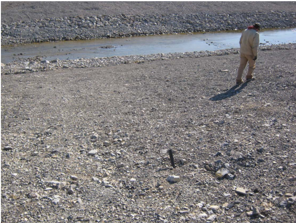
Photo 28, Garrow Lake Dam, West abutment, Breach slope from the crest
