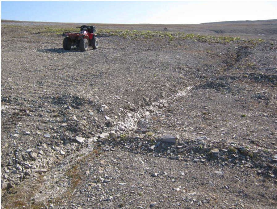
Photo 86, New Quarry, Top of South slope, Old tension crack healed with erosion
