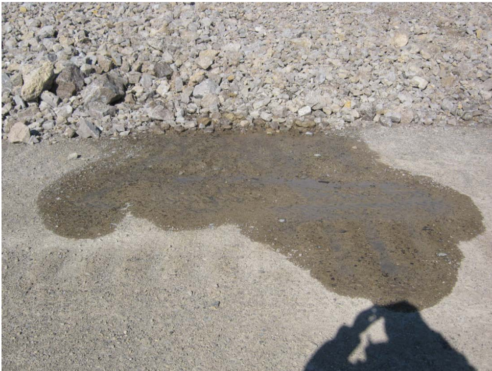
Photo 12, Operational Landfill, Northeast Toe, Minor thaw seepage (clear) at toe
