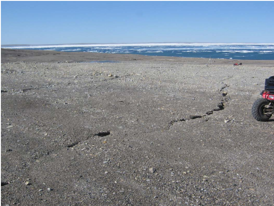
Photo 60, Subsidence Area, Central backfilled area, Two old tension cracks (~40m x 0.3m)
