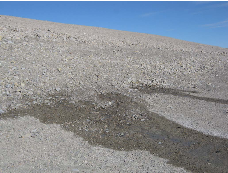
Photo 13, Operational Landfill, Central Toe, Facing Northwest across slope, Minor thaw seepage (clear) at toe
