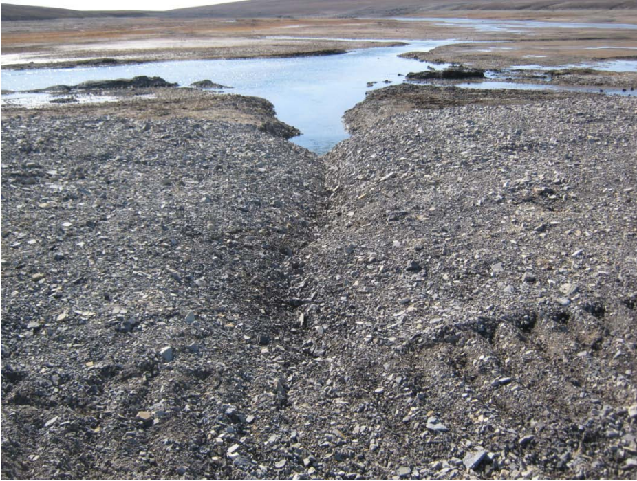
Photo 39, Garrow Lake, East end of Wave Break, Seepage/thaw settlement channel
