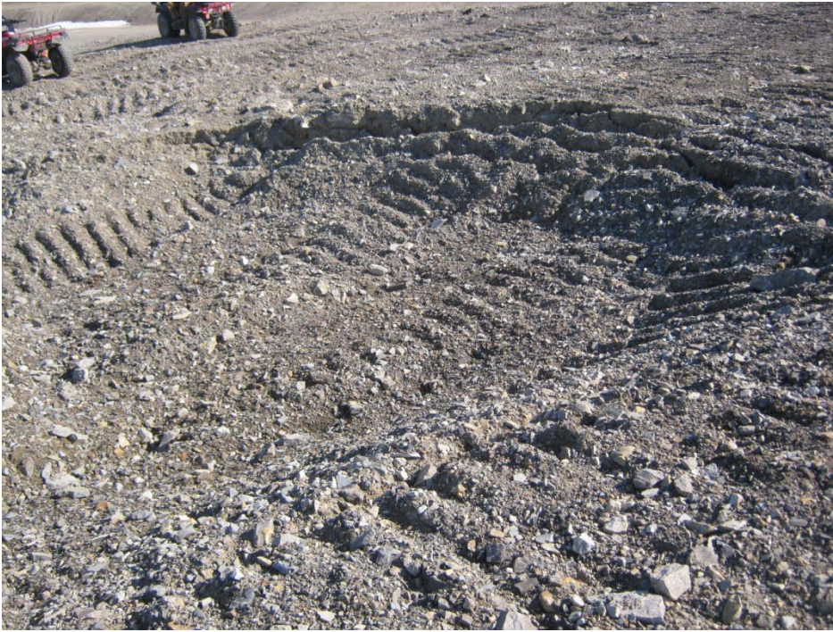
Photo 55, Subsidence Area, South end, Thaw settlement (~8m x 8m x 1m deep)
