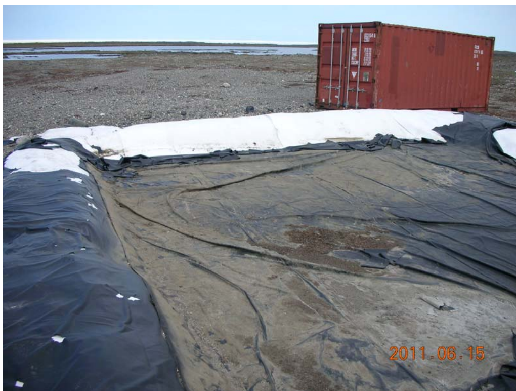
PICTURE 2: Empty Lagoon with Missing Liner
