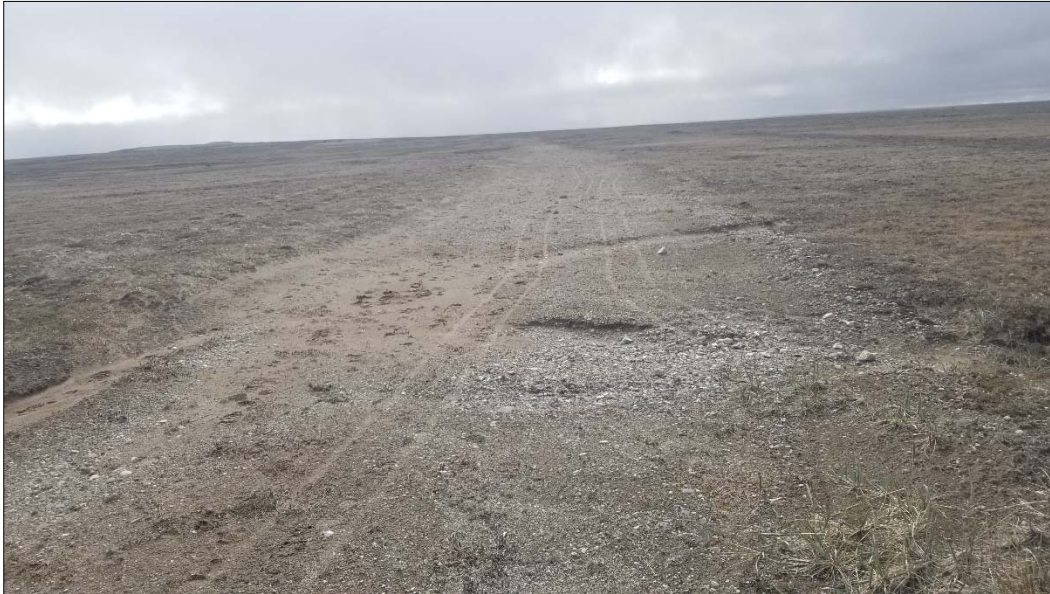
Photo 15 : Washout on Access Road to Main Station Area, Viewpoint 127
