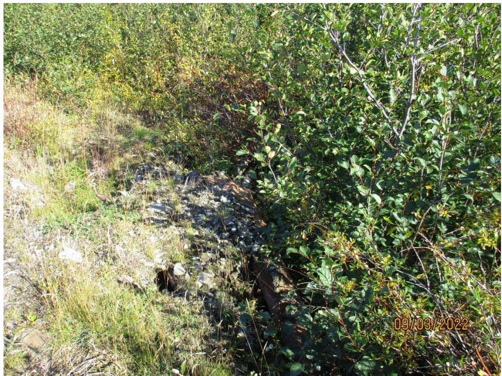
Photo 18: Quarry Pit main subsidence area looking east.
