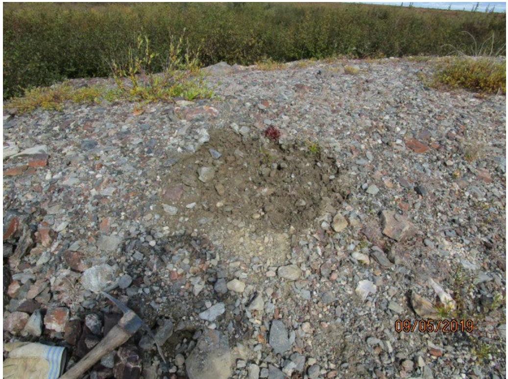
Photo 13: Small area of subsidence at B-zone Vent Raise in 2019 after filling.
