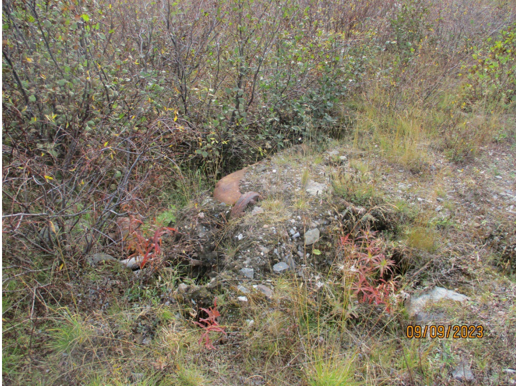
Photo 17: Quarry Pit main subsidence area – no change from previous years.
