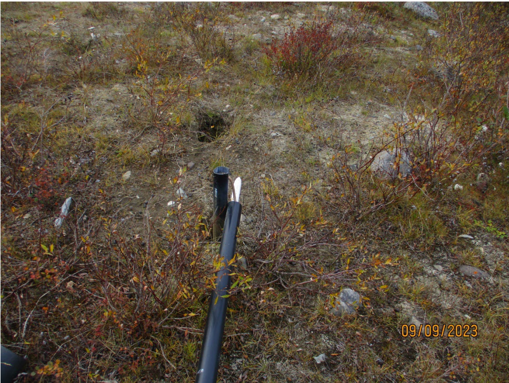
Photo 18: Thermistor T-2 casing damage unchanged from last year.
