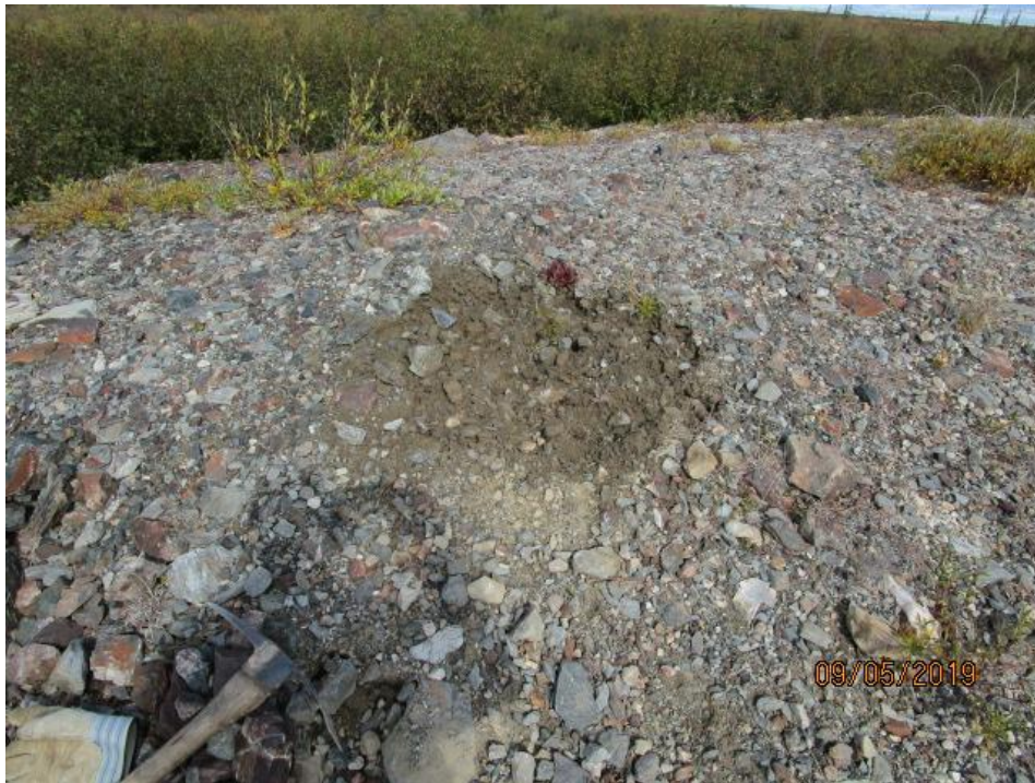
Photo 10: Small area of subsidence at B-zone Vent Raise in 2019 after filling.
