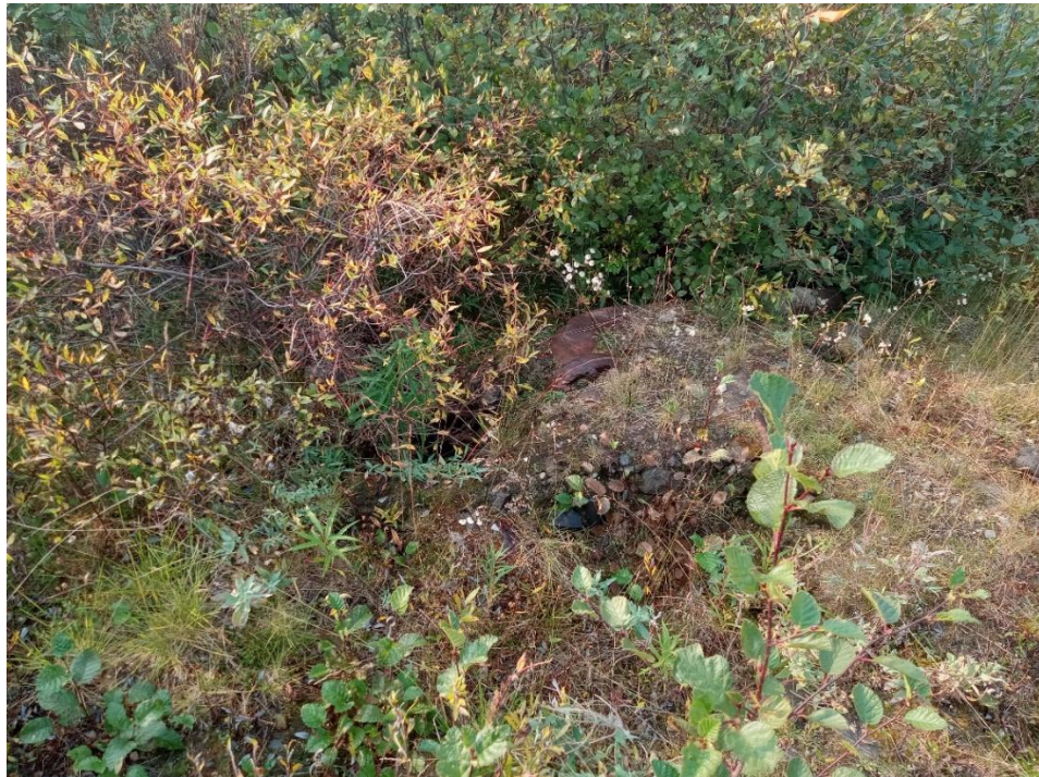
Photo 14: Quarry Pit main subsidence area – no change from previous years.
