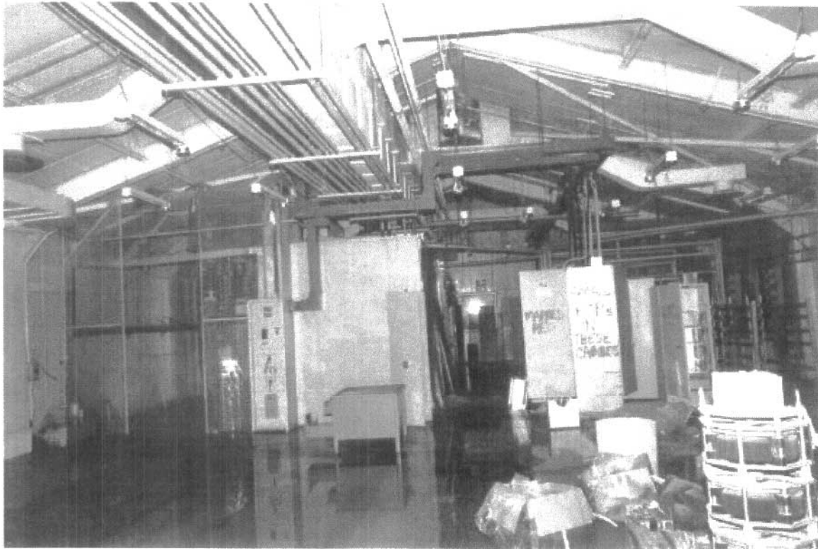
Photo 29 – Power/Equipment Building interior on Aug. 3/97
