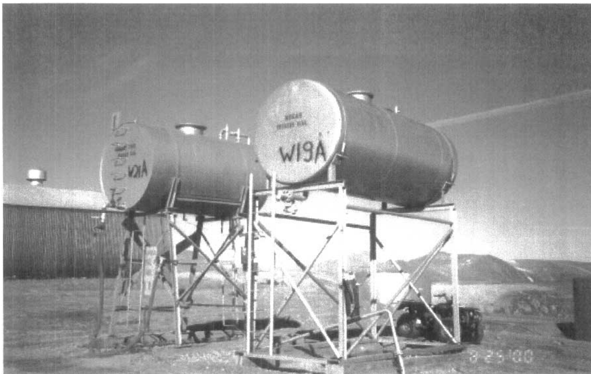
Photo 18 – Mogas and Fuel Tanks
