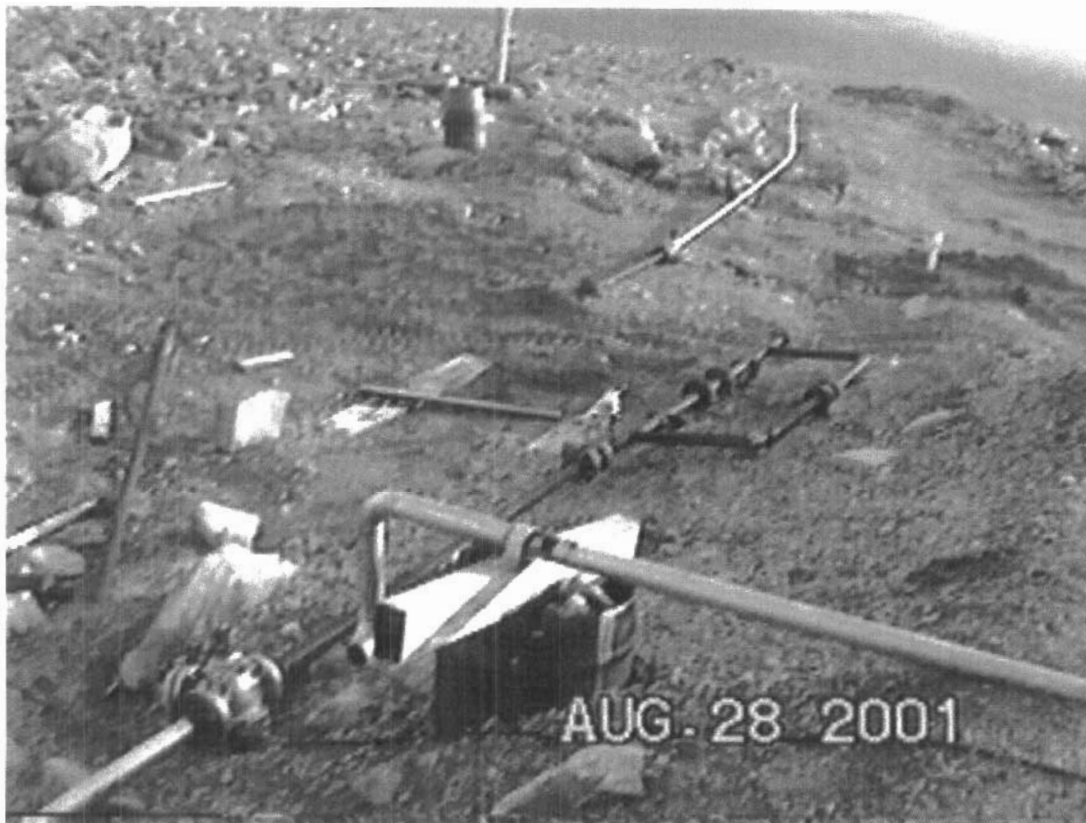
Photo 62 – Debris Area No. 34 (Dwg. 150)
