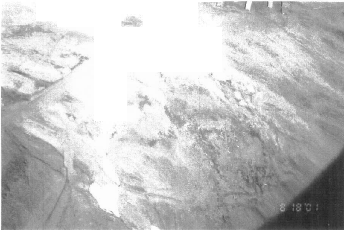
Photo 78 – Debris Area No. 50 (Dwg. 164)
