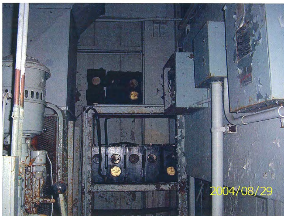
Photo 54 Batteries in Generator Room - Garage
