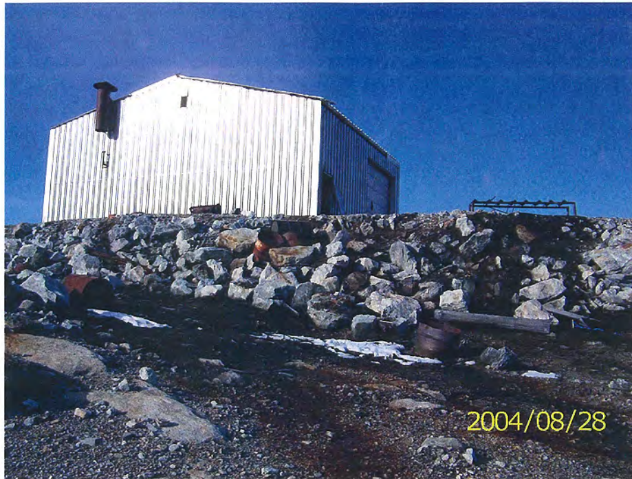
Photo 33 Staining below Garage, looking north
