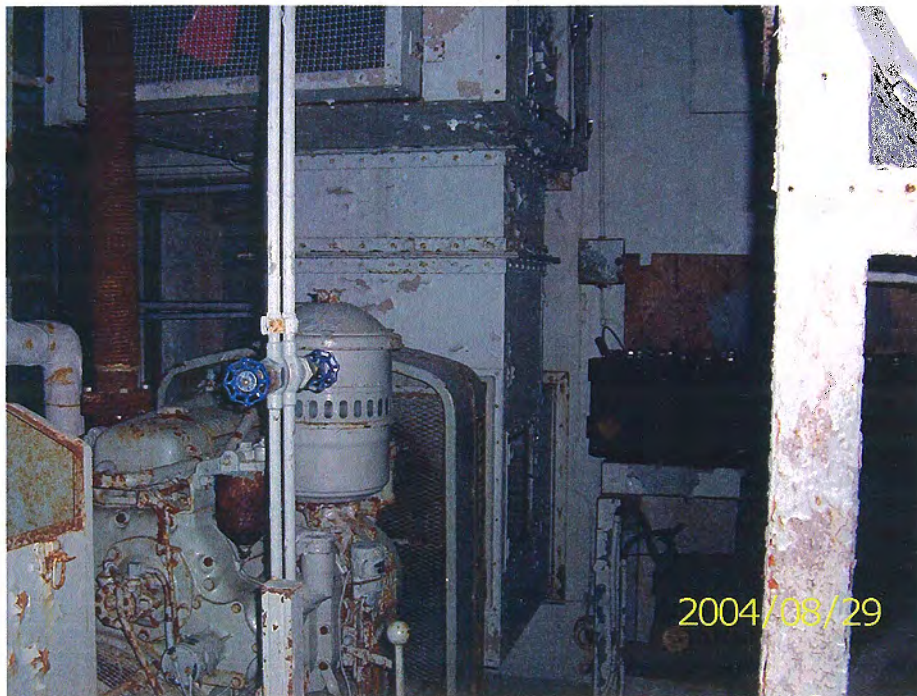
Photo 50 Genset - Module Train
