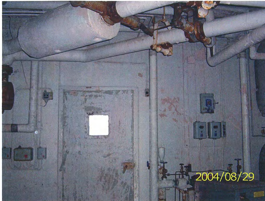
Photo 51 Typical piping in Warehouse
