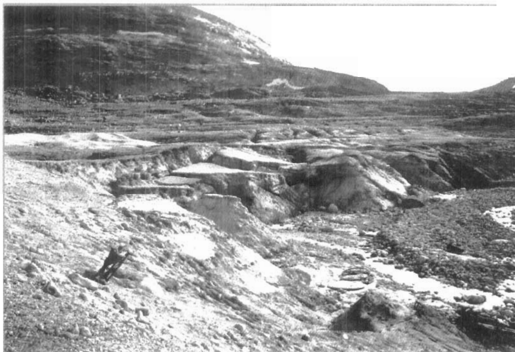
Photo 4 - Major Washout near Intersection
