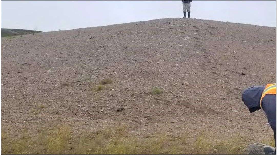
Photo 1: Small Depression at Northeast Corner of NHL, Viewpoint 94
