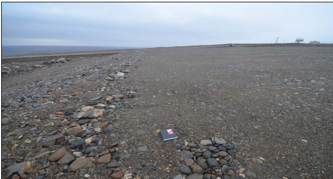
Figure 10: Photo - 2013-F3-NHWL-53 - Feature D - View W - of the discontinuous crack on the southern surface of the landfill - (new observation).
