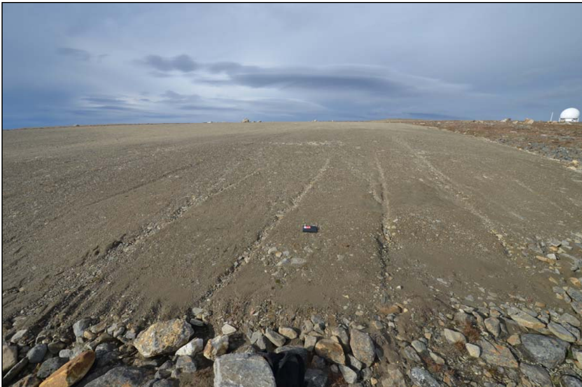
Figure 4: Photo - 2013-F3-SW-65 - Feature P - view N - of six erosion channels extending from the southwestern landfill surface to the toe taken from the bottom of channels, located on Lobe F - (previously observed).
