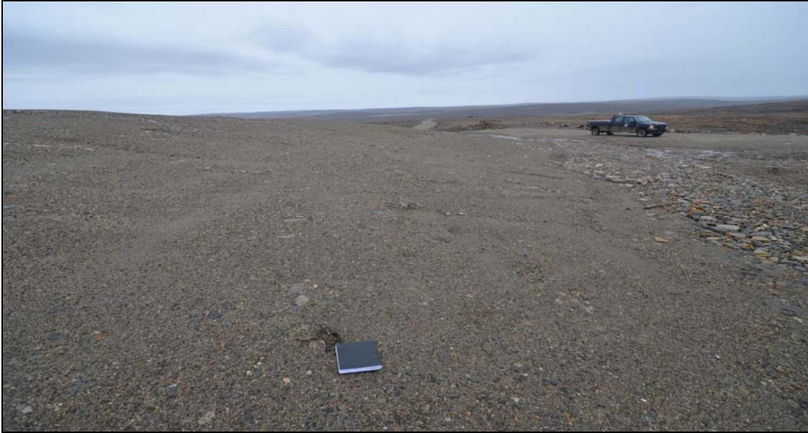
Figure 5: Photo - 2013-F3-W-9 - Feature A - View W - of 1 of 4 small depressions identified on the northern section of the landfill cap - (New observation).
