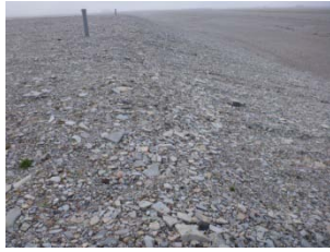
Photo B5 West view of differential settlement feature E on north crest and slope
