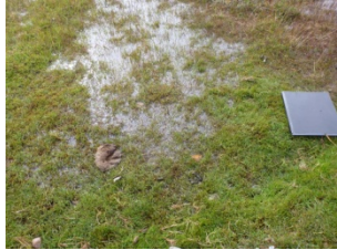
Photo G4 Close up view of water staining
