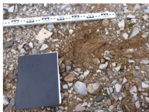
Photo F13 West view of exposed debris on toe of slope
