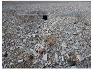
Photo B2 View of settlement feature B near southwest corner crest
