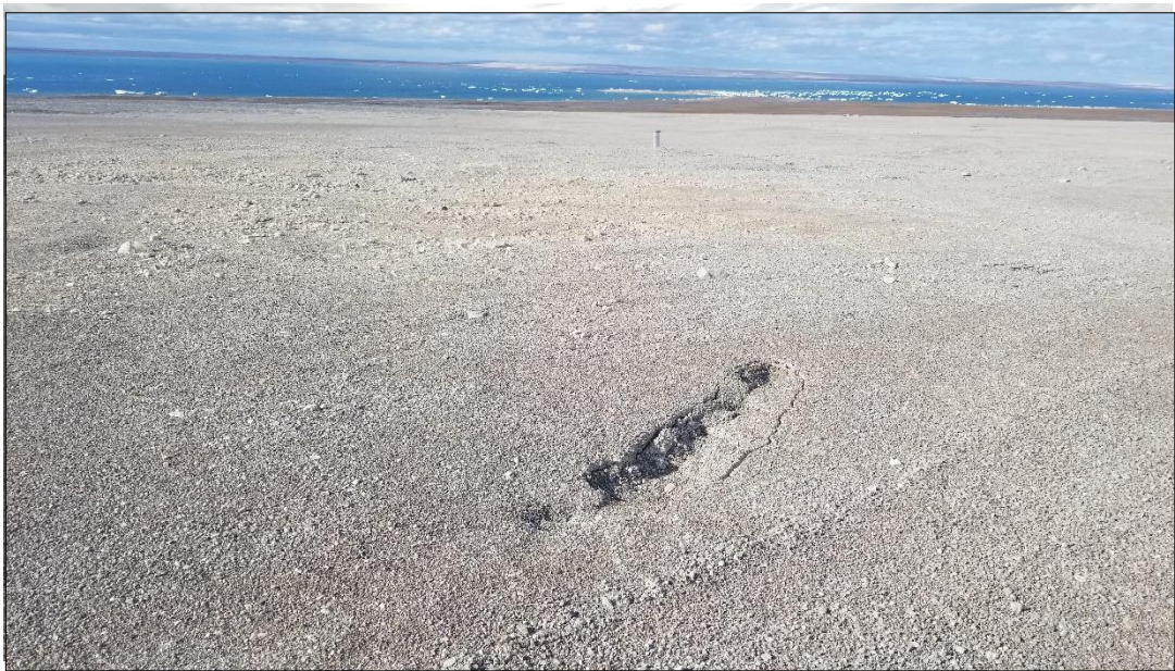
Photo 7: Small Crack West of Non-Hazardous Waste Landfill.
