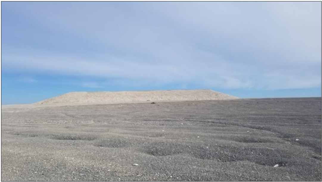
Photo 1: Erosion around the Tier II Landfill.
