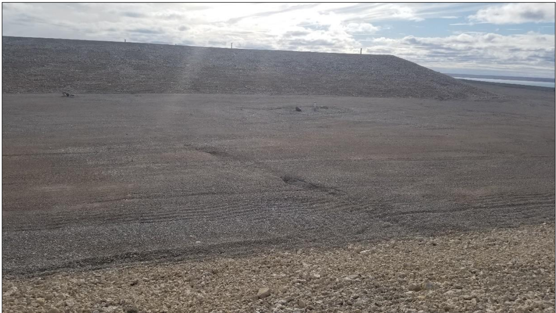
Photo 6: Crack adjacent to Non-Hazardous Waste Landfill.
