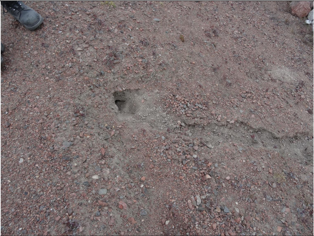
Description: Animal Burrow Holes found in the Berm Perimeter – View 2
