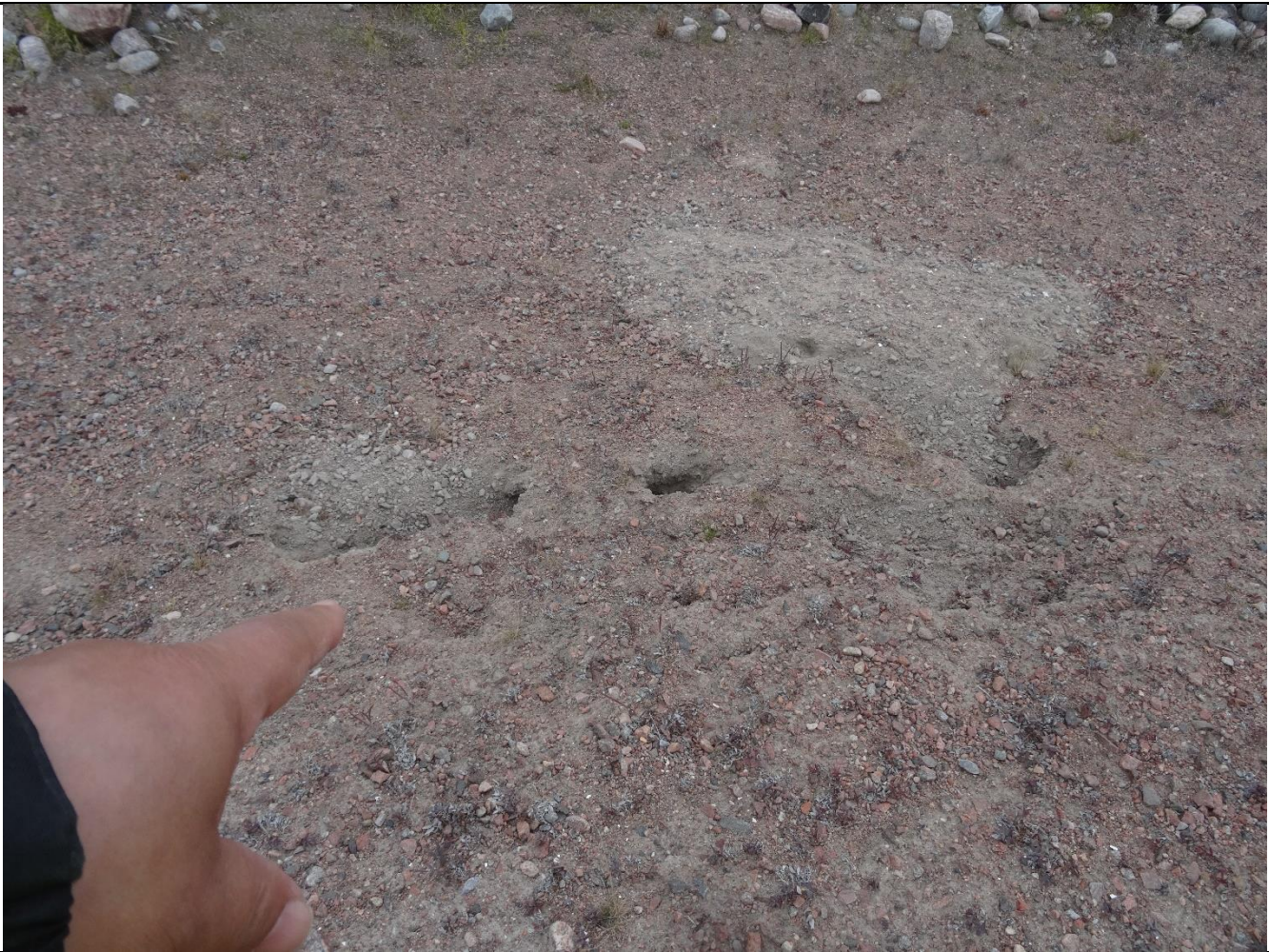
Description: Animal Burrow Holes found in the Berm Perimeter – View 1
