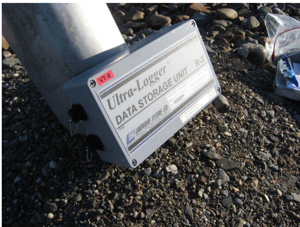
Photograph 127. VT-8 Data Logger (FOX-2 34). ↑
