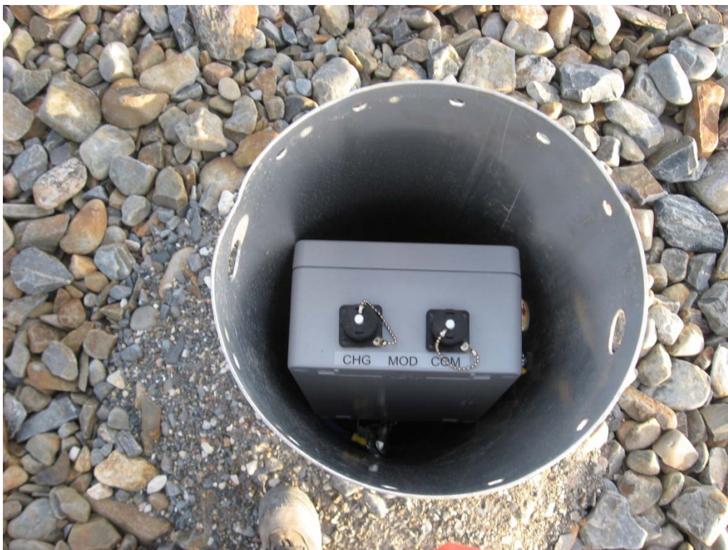
Photograph 118. VT-6 Data Logger (WP 110, FOX-2 25). ↑
