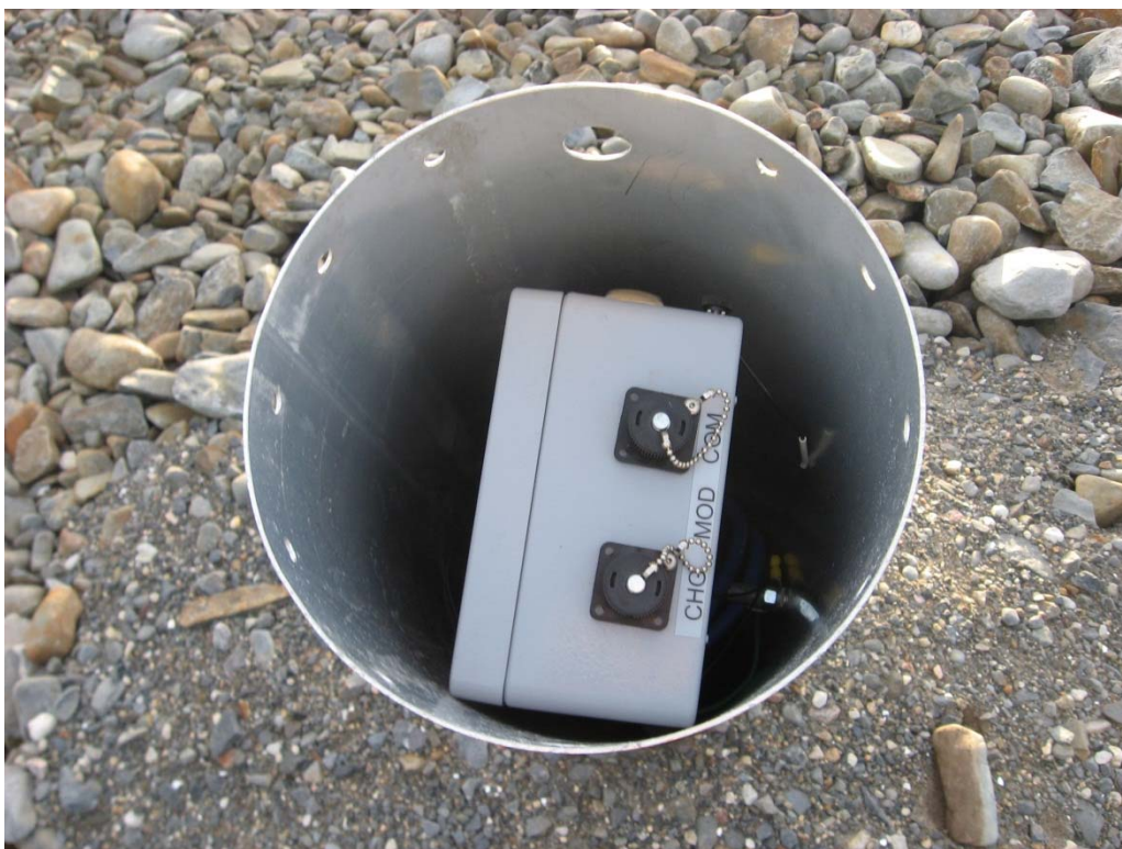
Photograph 119. VT-8 Data Logger (WP 111, FOX-2 26). ↑
