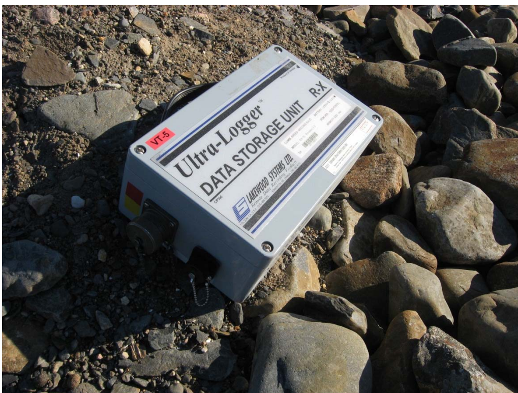
Photograph 123. VT-5 Data Logger (FOX-2 30). ↑
