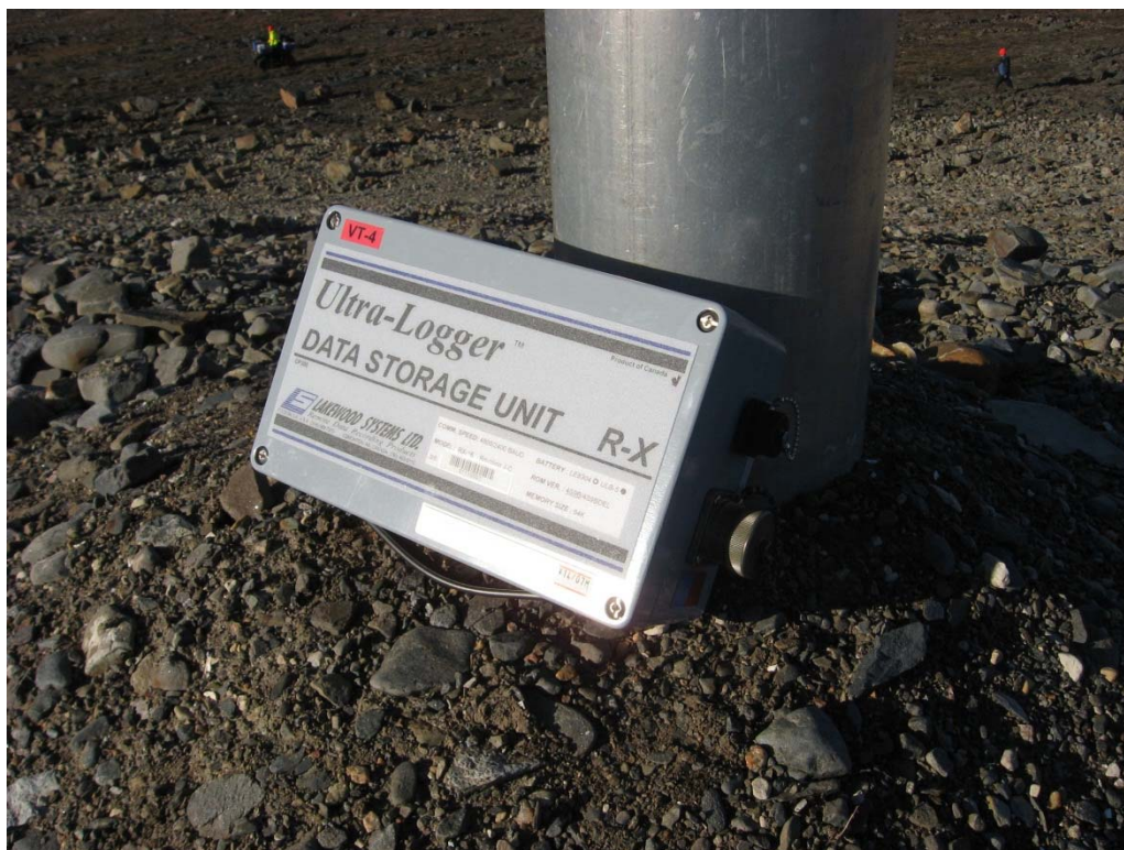
Photograph 65. VT-4 Data Logger (FOX-2 36). ↑
