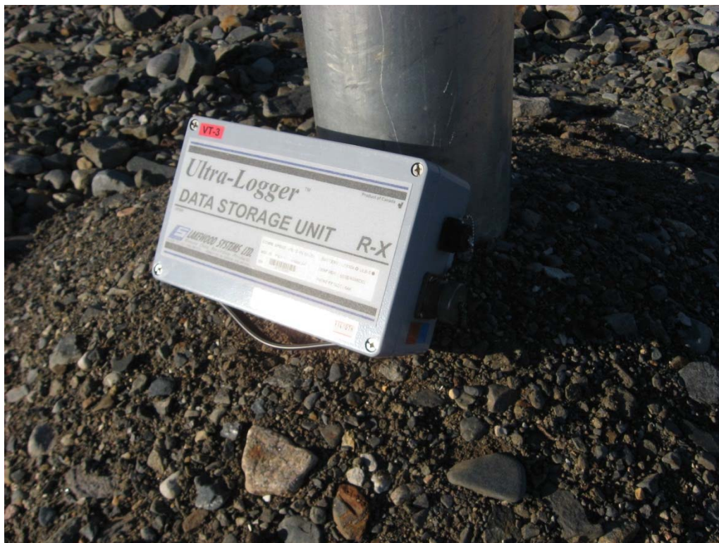
Photograph 68. VT-3 Data Logger (FOX-2 39). ↑
