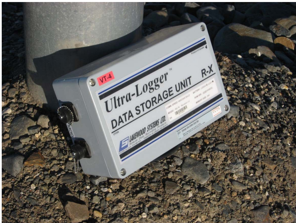
Photograph 66. VT-4 Data Logger (FOX-2 37). ↑
