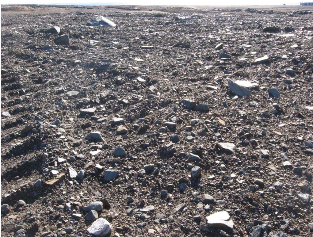
Photograph 12. Rough Finish Grading/Minor Settlement – Looking S (WP 153, FOX-2 134). ↑
