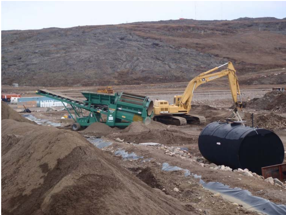
Water storage tank, screening Plant and excavator
