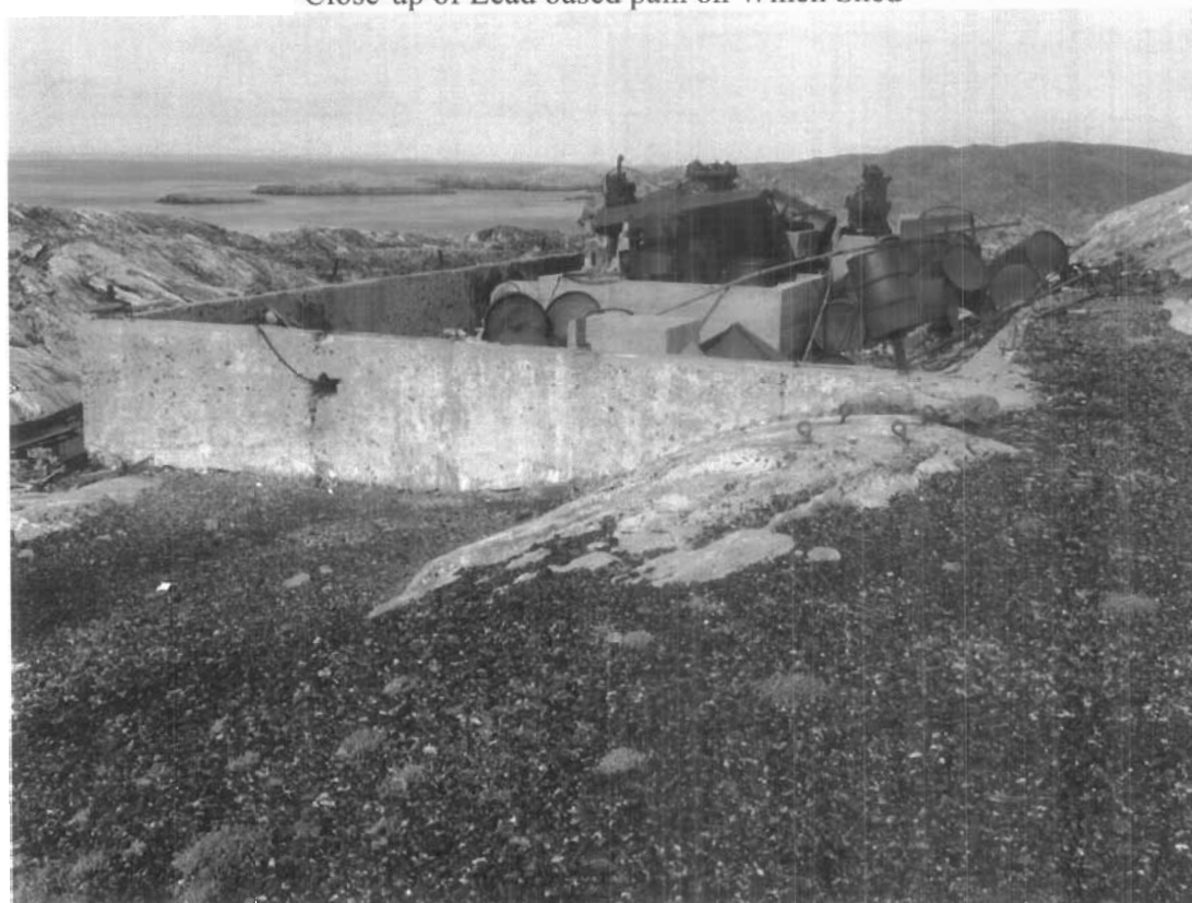
View of Generator Building Foundation and Debris
