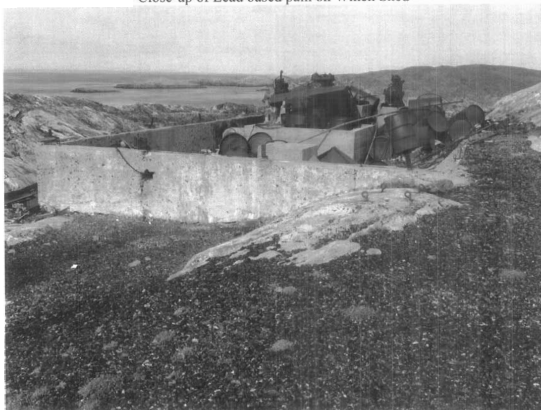
View of Generator Building Foundation and Debris
