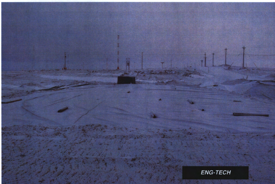
Photograph 6 – Ground heating system, in operation.
