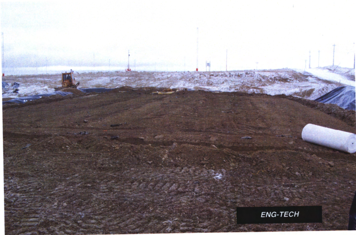
Photograph 3 – Area of ground heating system, without insulation cover.
