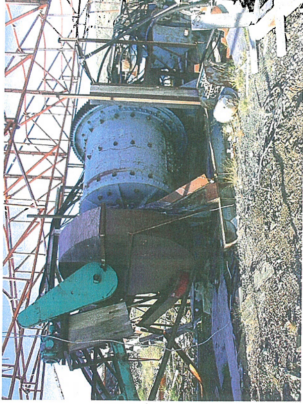
Photo 13: Ball mill inside Mill Building
