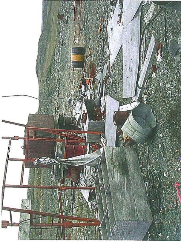
Photo 26: Flagging showing ET 1111 and debris inside Garage,
