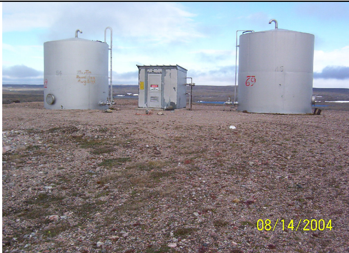
Photo 11: POL tanks view northwest.
