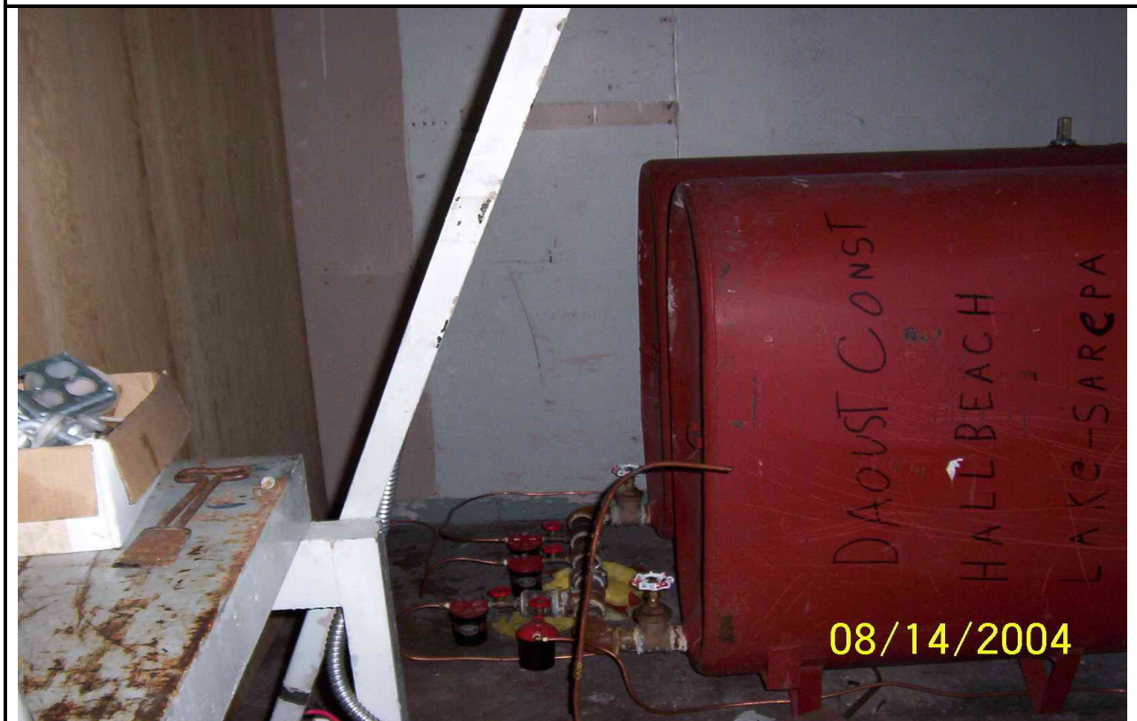
Photo 2: Module Station, fuel tanks inside generator room.
