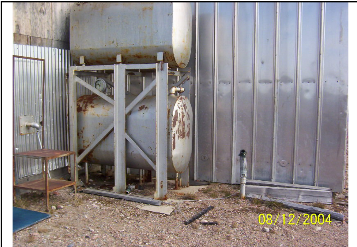
Photo 5: Warehouse fuel tanks.
