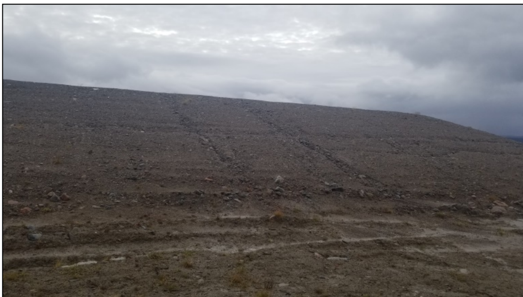
Photo 4: Erosion channels on NE corner.
