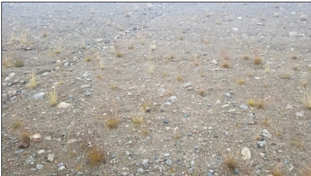
Photo 3: Erosion on NE corner of landfill.
