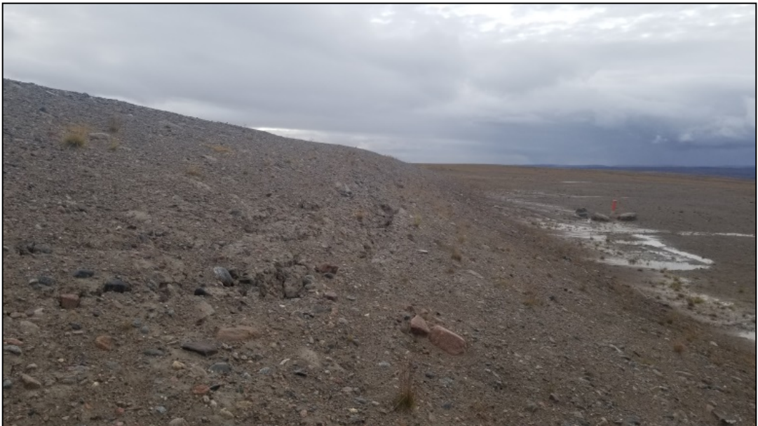
Photo 8: Frost crack looking west on the north side of the landfill.
