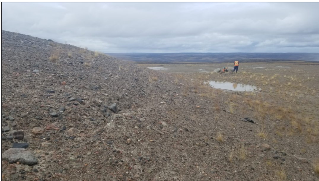
Photo 5: Frost crack on the southern side of the landfill.
