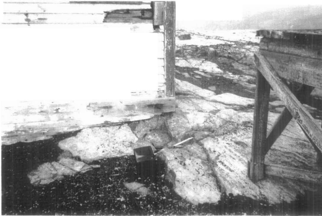
Photo 2.21 Facing south at main house where lead paint sample RI-41 was obtained.
