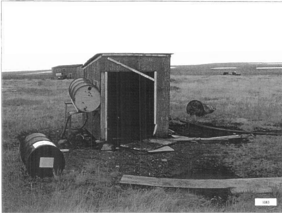
Generator building - note contaminated soil.
