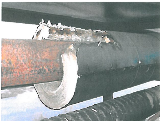
Photo 3: Close-up of asbestos pipe wrap
