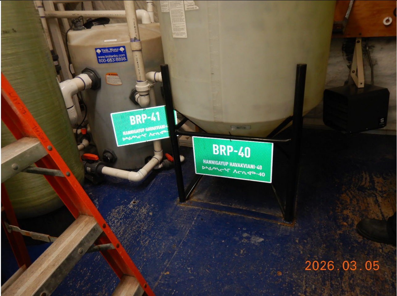
Description: Inside reverse osmosis plant at MLA. Note signs for monitoring.
