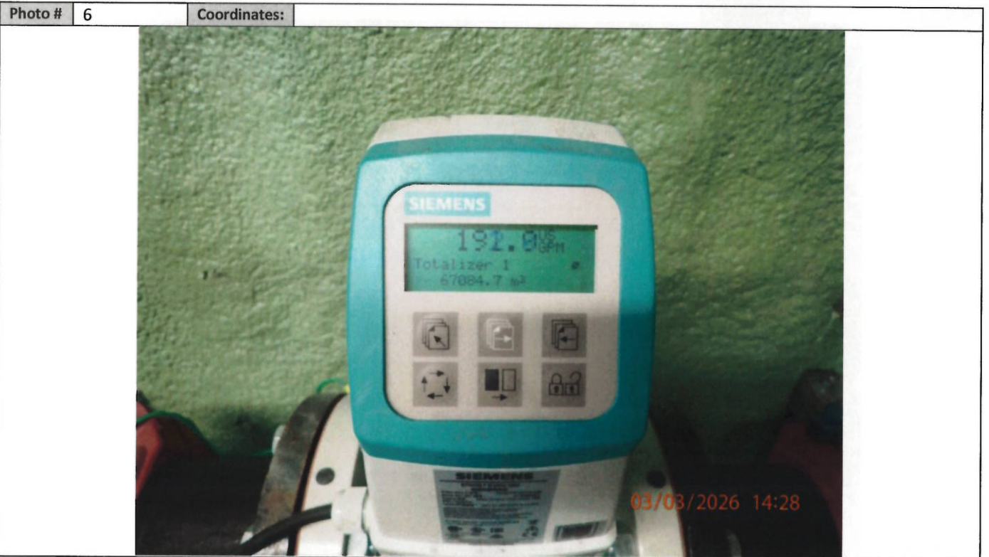
Description: Water meter inside the main water supply seacan.
