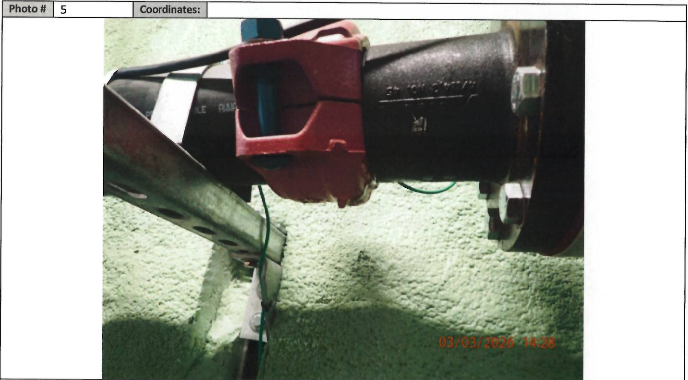
Description: Water leak from the main water line in the main water supply seacan.
