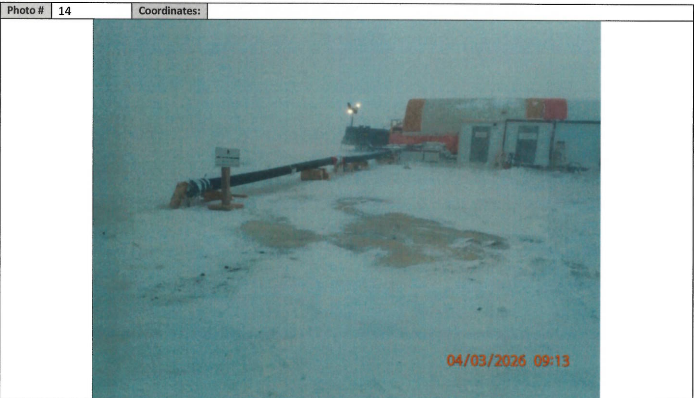
Description: Grey water discharge location at goose forward. The release flows right onto the PAD of the camp.
