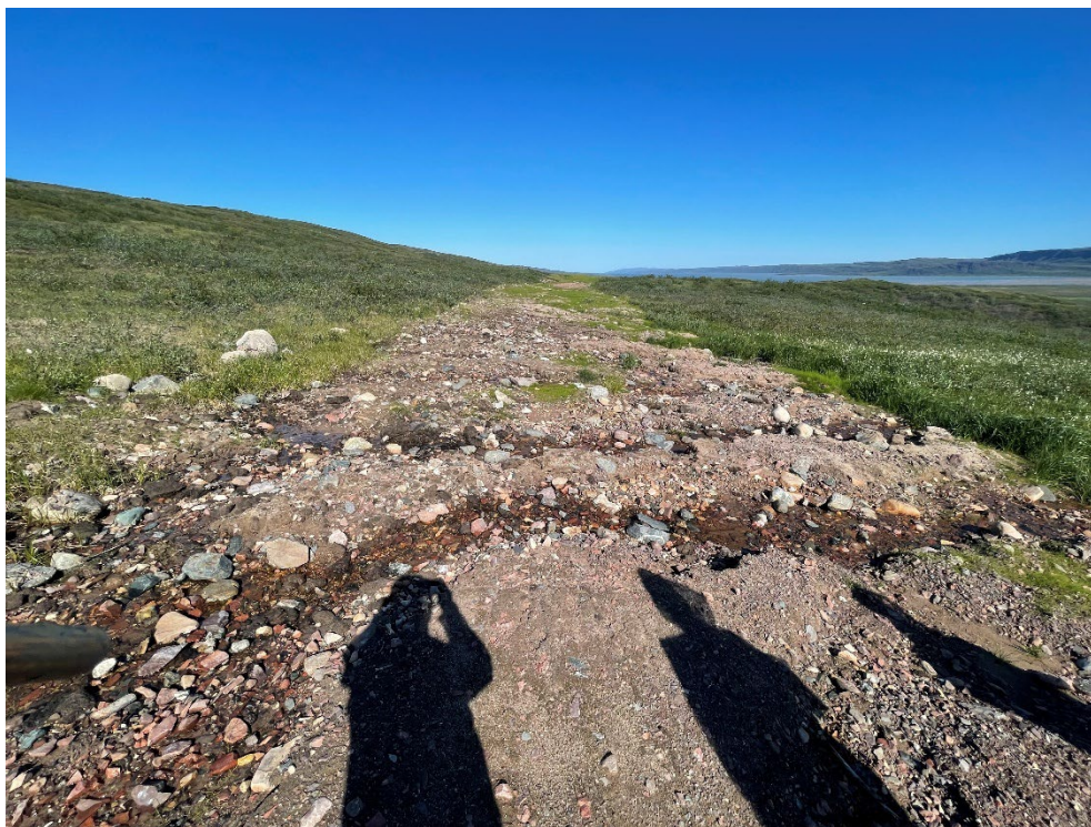
Photo 1: Surface Drainage Observed on WIR Route during Summer 2024 Survey
