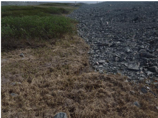
Seep at d/s toe. Water quality sample collected
