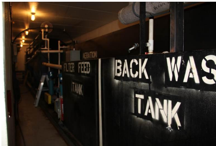
Photo 43: Inside the sewage treatment plant
