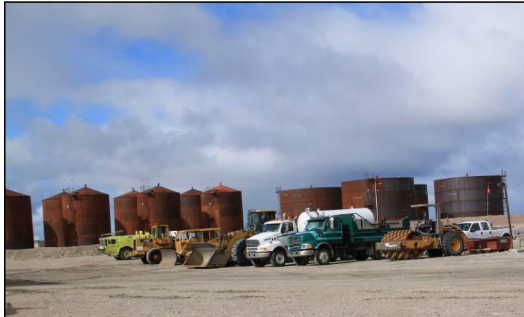
Photo 24: Main tank fuel farm
