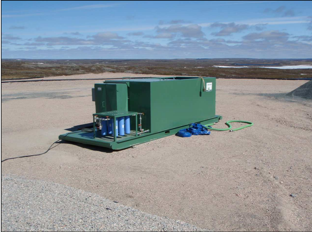
Photo 10 – Oztec Water Remediation Unit
