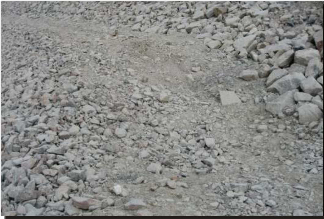
Photo H.4 C1 Diversion Channel - Reach A: Settled fill in Reach A on berm.
