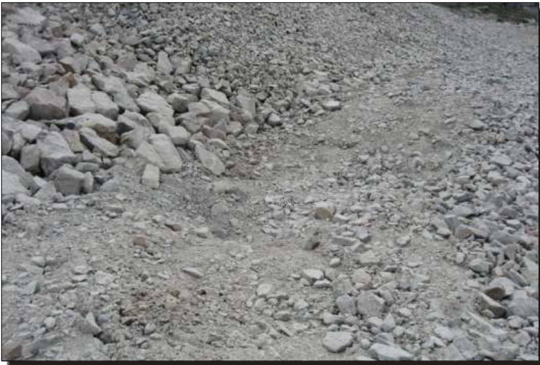
Photo H.6 C1 Diversion Channel - Reach A: Settled fill.
