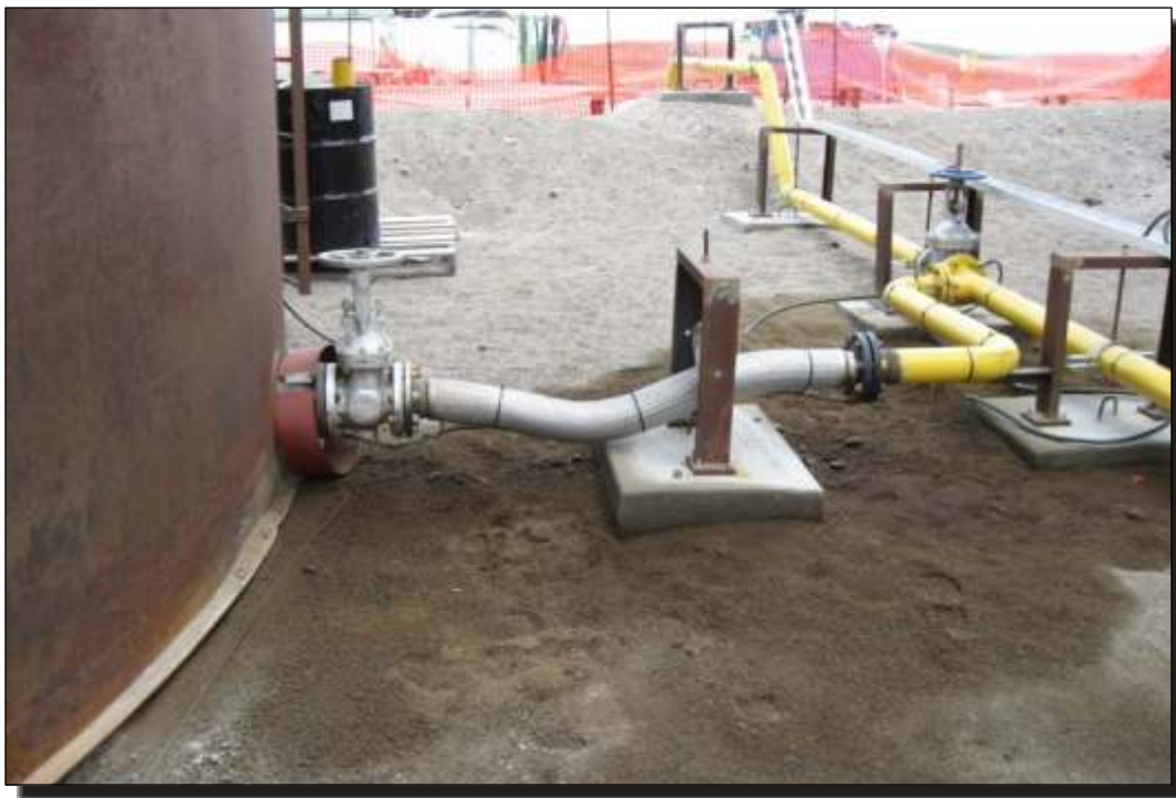
Photo D.6 Phase 1 Tankfarm: New flex connections (photo taken at Tank 5).
