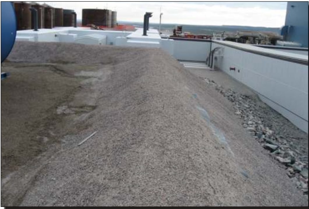
Photo G.4 Generator Tank: East Berm. Exposed liner.
