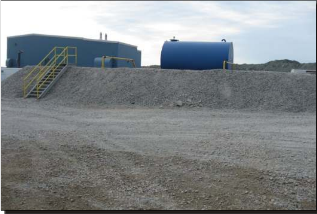
Photo G.1 Generator Tank and Containment berm.
