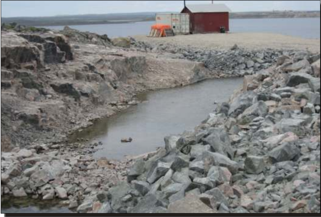
Photo H.7 C1 Diversion Channel - Reach A: Outlet. Ponded water.
