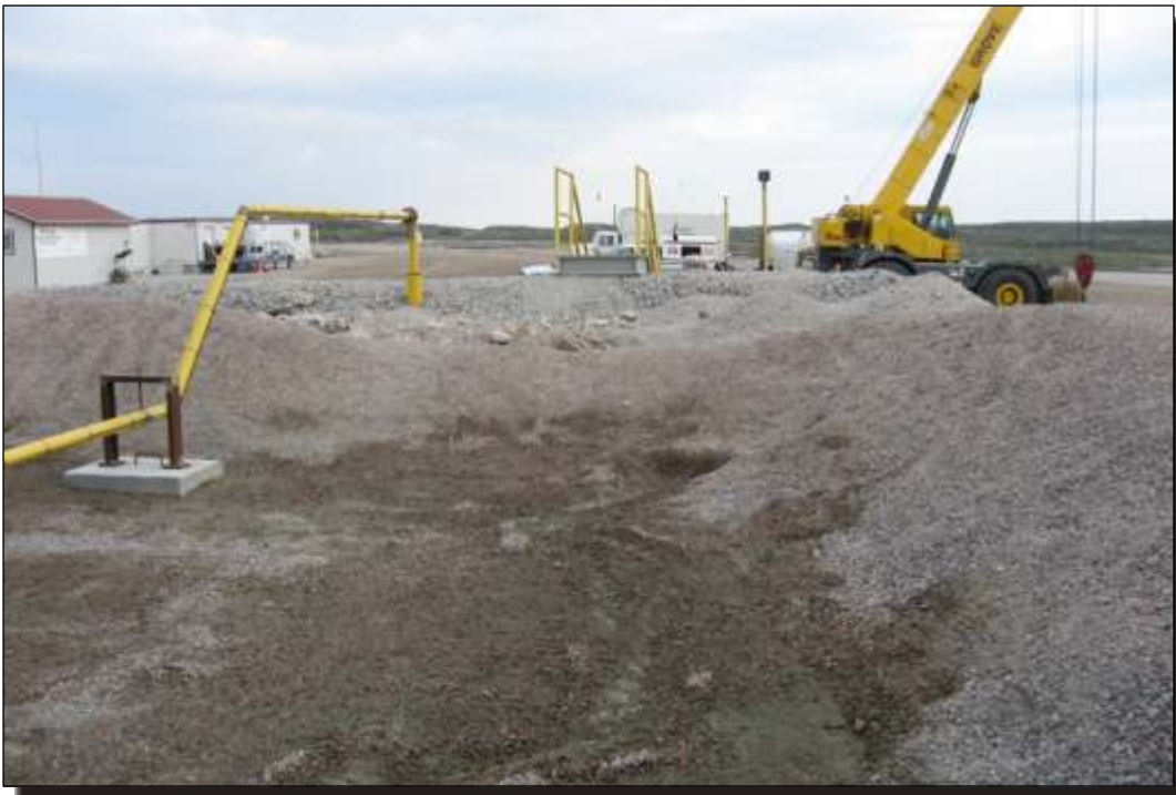
Photo G.2 Generator Tank: Low spot in West Berm.
