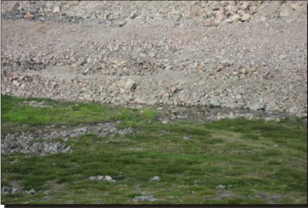
Photo C.4 East Dam: Downstream slope. Ponded water and dam toe.
