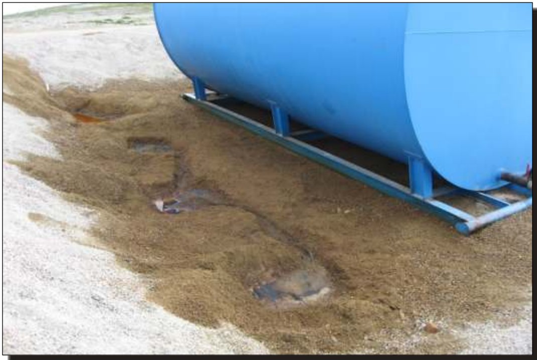
Photo F.2 Airstrip Fuel Tank: Stained area, exposed liner.
