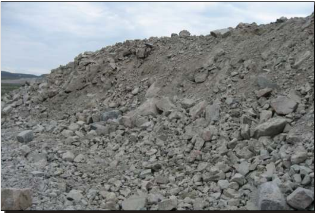
Photo H.18 C1 Diversion - South Berm. Pit Perimeter Road. Slough in road fill.
