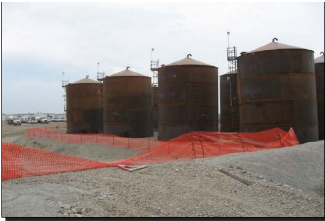
Photo D.1 Phase 1 Tankfarm: Eight 500,000 litre tanks, looking southwest.
