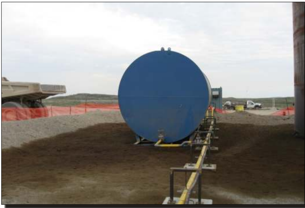
Photo D.7 Phase 1 Tankfarm: 64,000 litre tank. Stained soil in tankfarm base.
