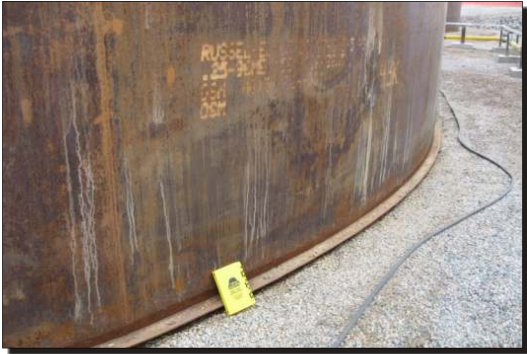
Photo D.9 Phase 2 Tankfarm: Tank 9 settlement under tank edge.
