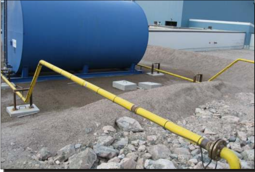
Photo G.3 Generator Tank: Stain in bottom of containment area.
