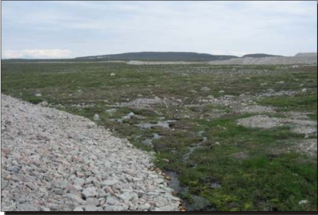
Photo H.13 C1 Diversion Channel - Reach C: Outlet. Ponded water.
