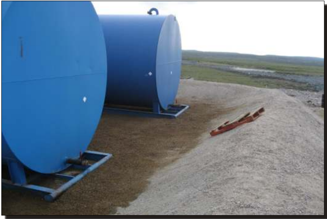
Photo F.3 Airstrip Fuel Tank: Stained area within tank farm.
