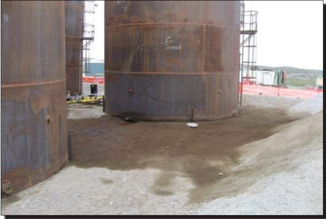
Photo D.3 Phase 1 Tankfarm: Stained soil adjacent Tank 7.
