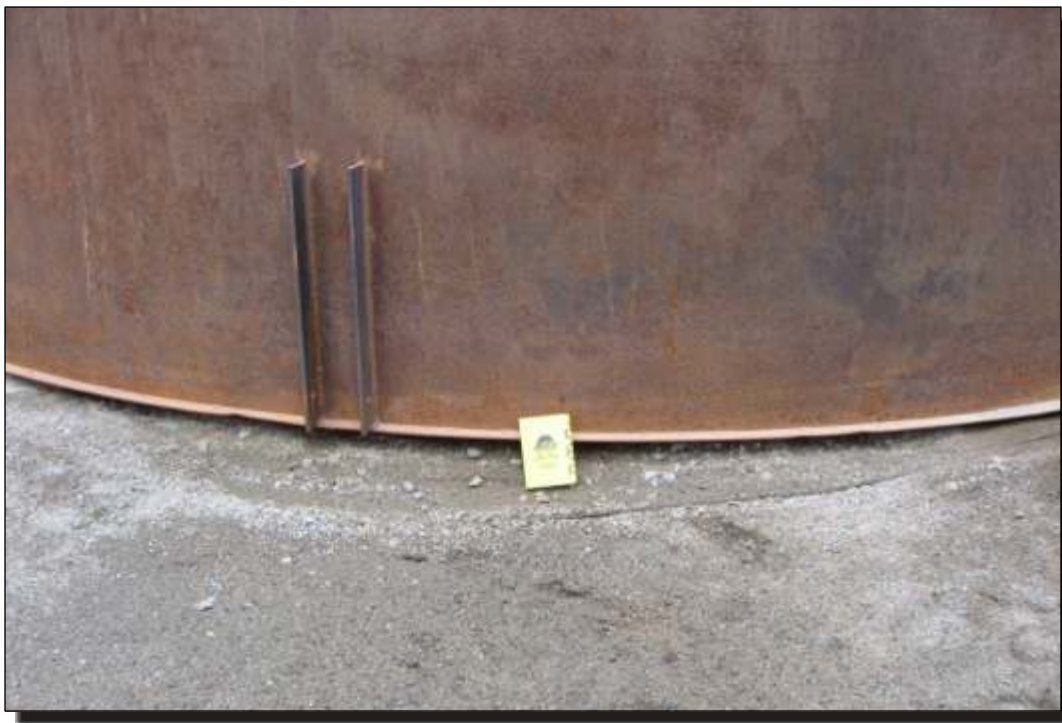
Photo D.2 Phase 1 Tankfarm: Tank 5. Settlement under tank edge.
