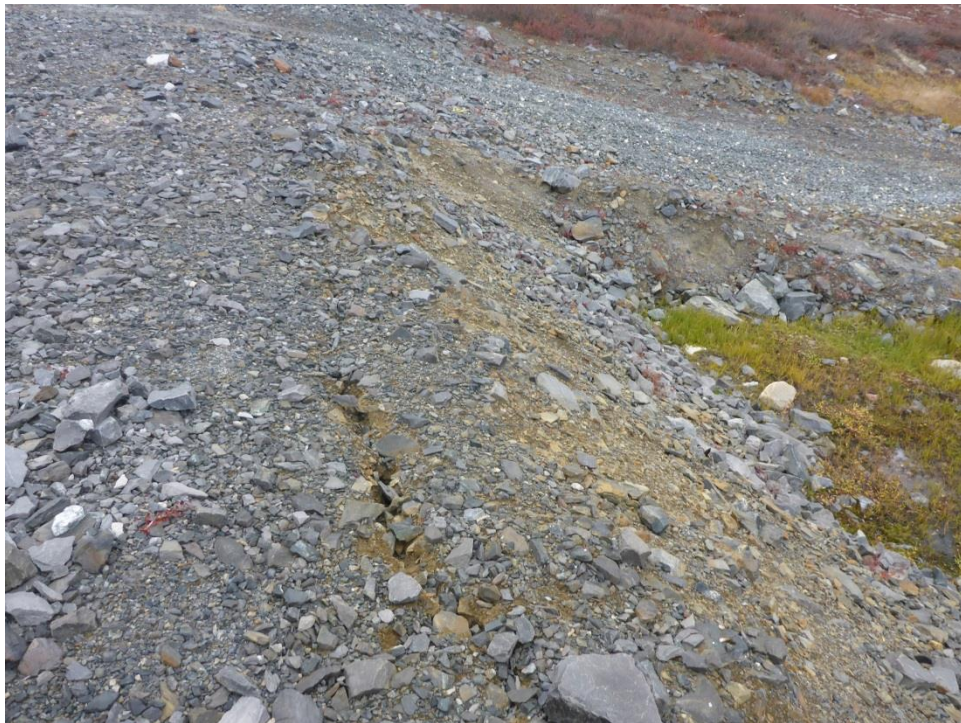
Photo 4: Close up view of the tension cracks in Lower Sewage Dam near the north abutment.
