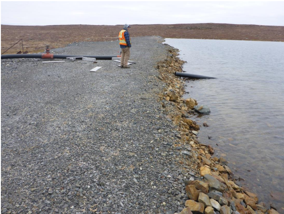
Photo 5: Looking southwest at the erosion in upstream face of Lower Sewage Dam.
