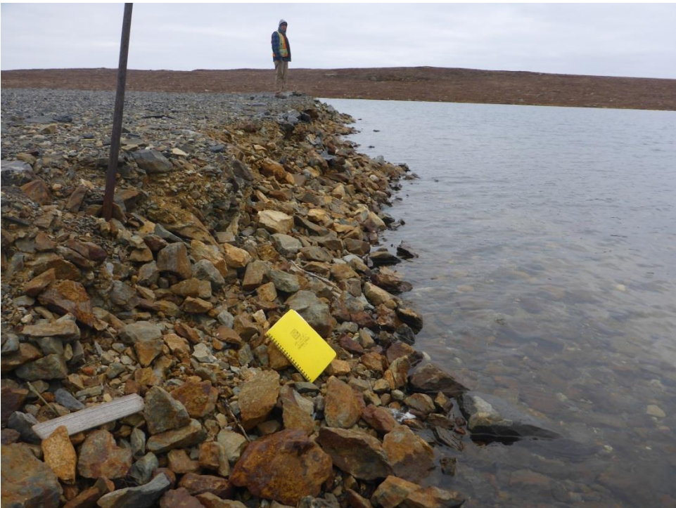
Photo 6: Close up view of the upstream face erosion in the Lower Sewage Dam.
