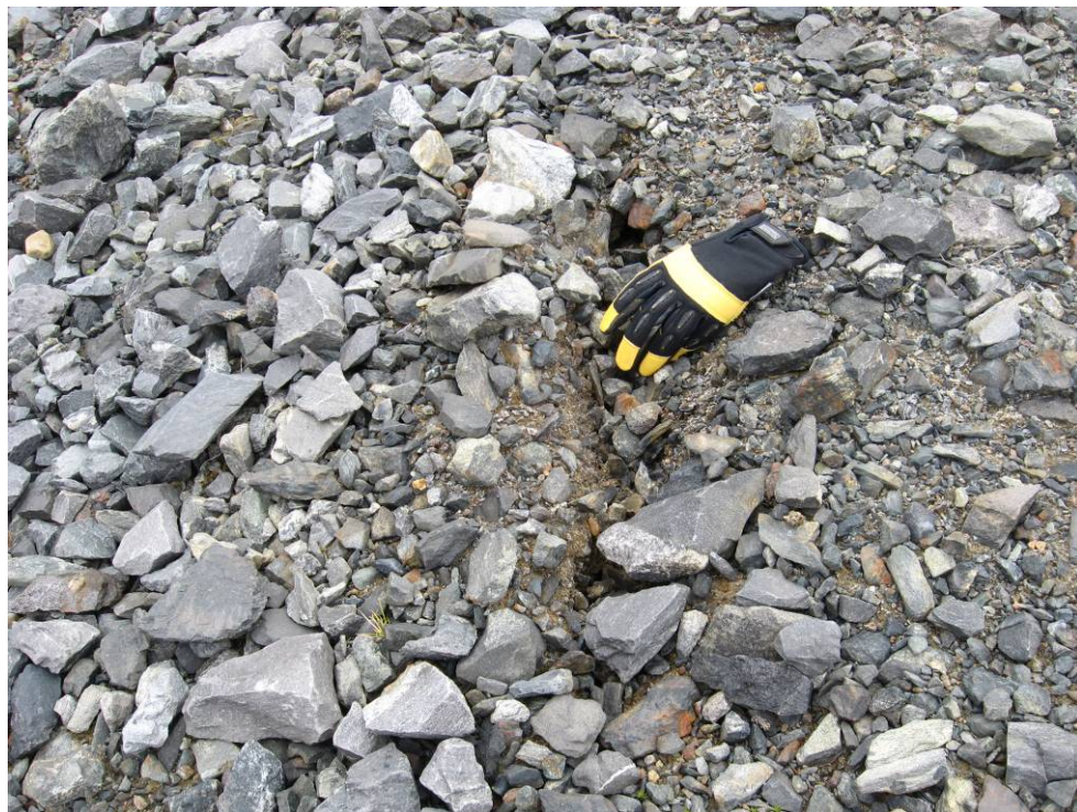
Dam 1C: Upstream-Minor Cracking
