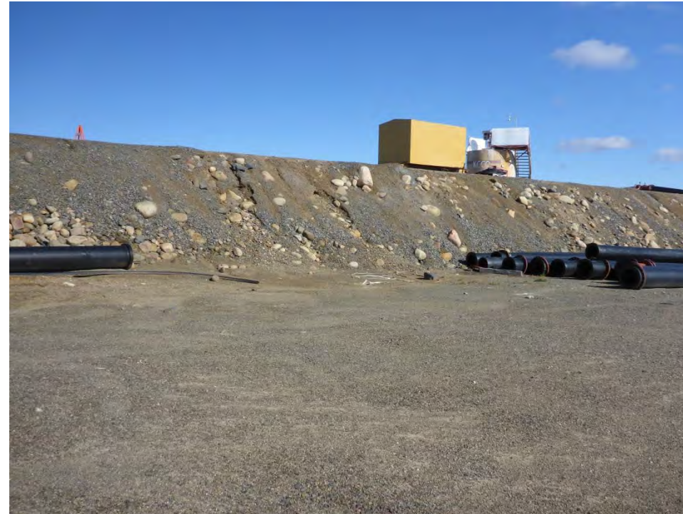
Photo 5: Downstream surface erosion of Dam 1A
