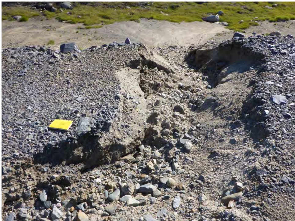
Photo 21: Close up of erosion gully in Dam 4.
