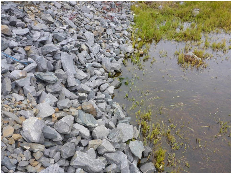
Photo 9: Looking at the seepage in the downstream toe in the north abutment of the Lower Sewage Dam.
