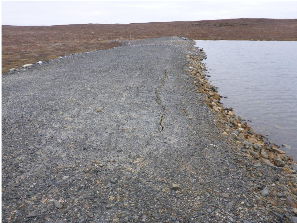
Photo 7: Looking southwest at the tension crack in the upstream portion of the Lower Sewage Dam toward the south abutment.
