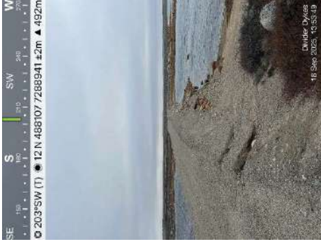
Photo 50: South Divider Dyke erosional feature on the upstream crest and embankment.
