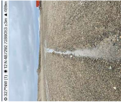
Photo 37: Minor swale conveying surface water over the Cell 4 NW corner esker cover.
