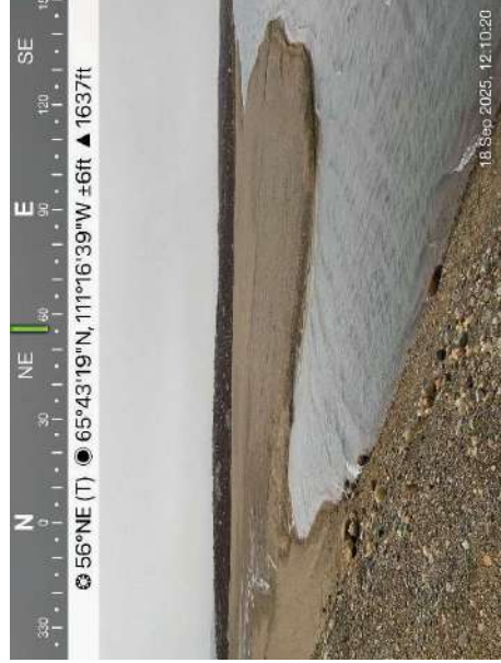
Photo 38: Cell 4 NW corner esker cover. Showing the minor swale conveying surface water, and some ponded water.
