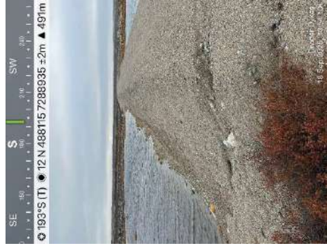
Photo 49: South Divider Dyke erosional feature on the downstream crest and embankment.
