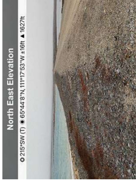
Photo 11: Dam 2 crest and upstream embankment, and Pond 2. Taken from the northern abutment.
