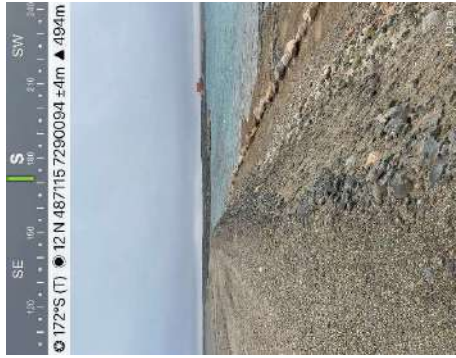
Photo 39: M Dam crest and downstream embankment. Taken from the M Dam crest near N Dam.
