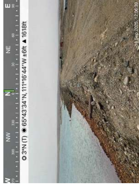
Photo 31: J Dam downstream crest and embankment. Showing Pond 2 to the west of the dam.
