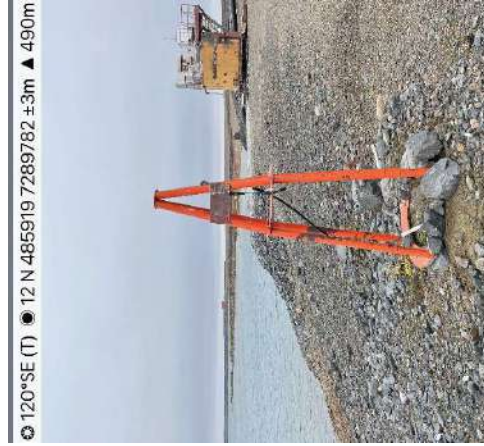
Photo 4: Thermistor D1A-00-01, installed on the crest near the northwest abutment.
