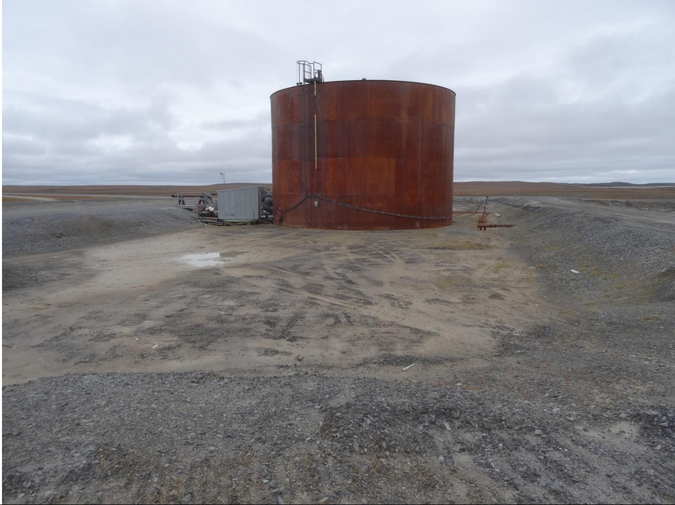
Description: Jet-A Tank Farm
