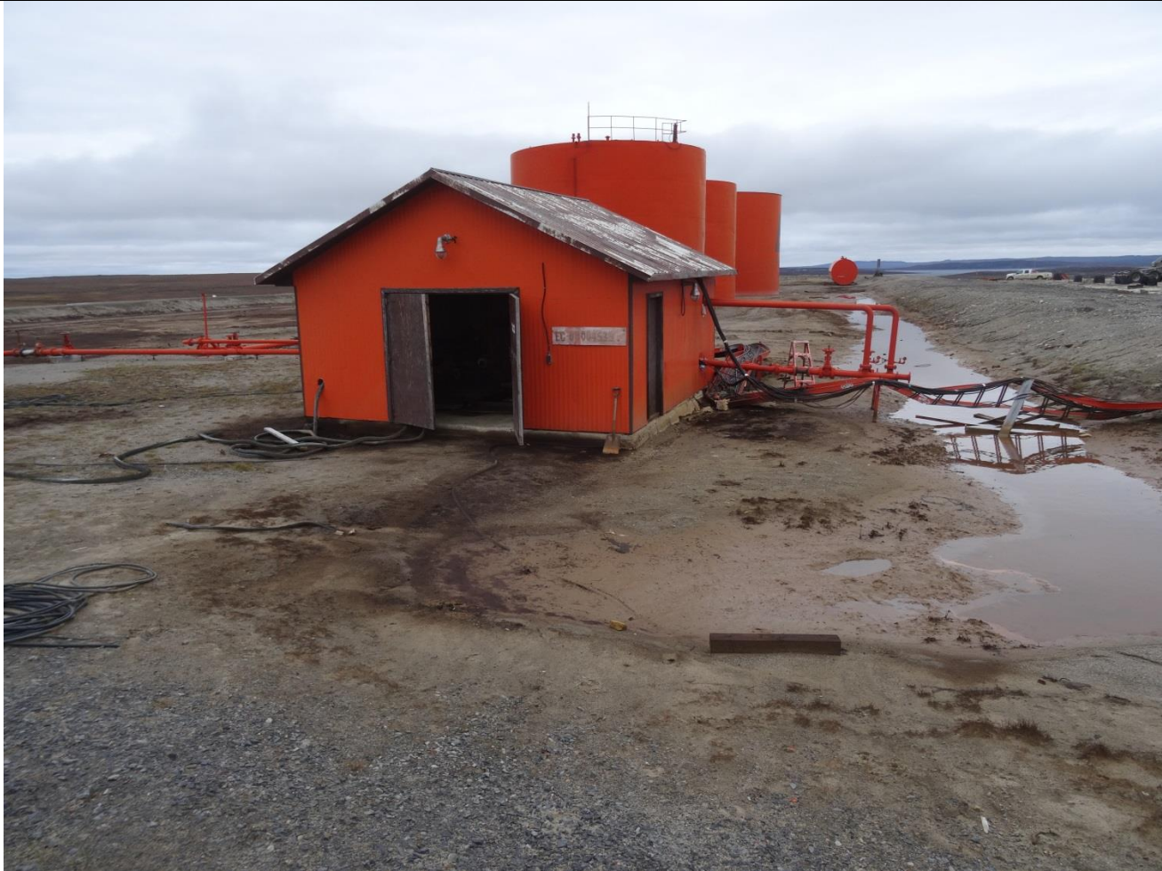
Description: Main Tank Farm – View 3 – Showing Pump Shack
