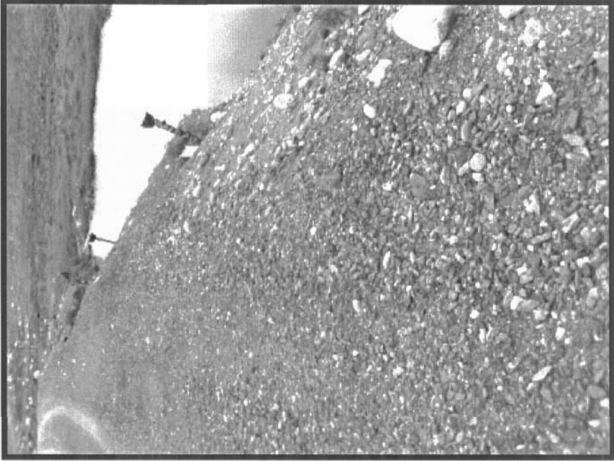
Photo 78 shows some minor cracking and minor settlement within the dark grey angular rockfill placed at the crest edge. This is a result of the relatively oversteepened toe directly proximal to the valve locations.
