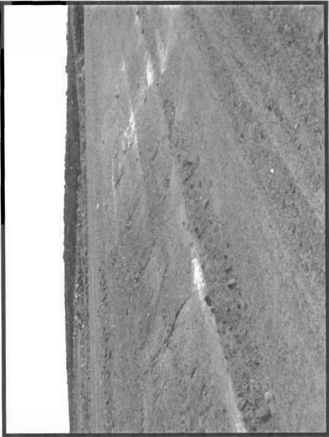
Photo 94 shows some minor erosional gullies on the downstream face.
