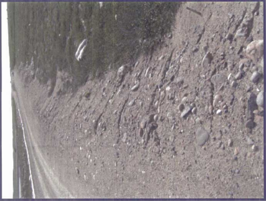
Photo 33 shows some minor erosional gullies located on the downstream side of Dam 5.
