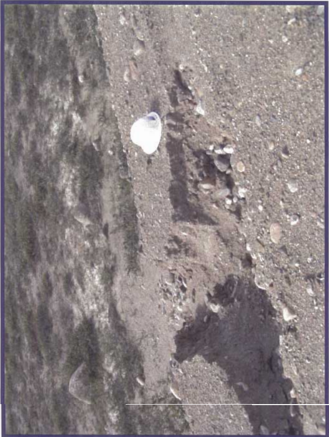
Photo 34 shows a significant erosional gully right in the middle of the downstream face. This gully should be repaired.
