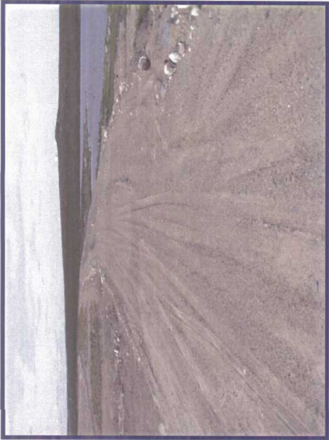
Photo 97 shows a shot of Dam 3 looking towards the north. The erosional gully noted here last year has been graded over and some changes to the crest have been made at the top of this reclaimed area.
