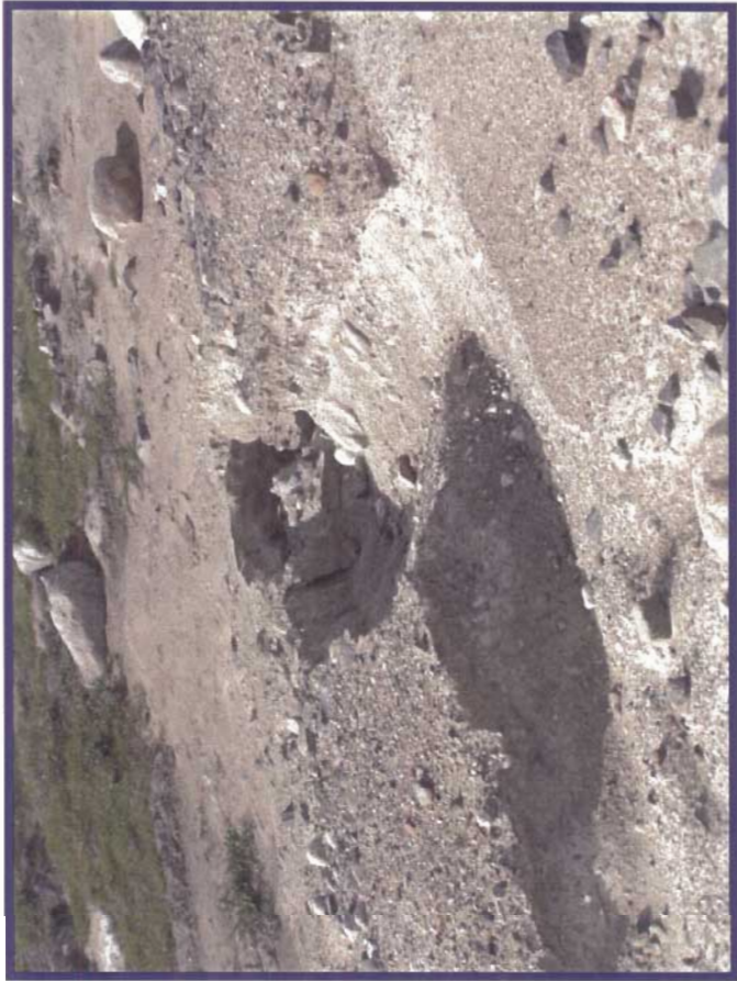
Photo 13 shows an erosional gully on the downstream face. This gully is located approximately 8 to 10 metres west of Thermistor 4-1. This gully should be backfilled to prevent any further erosion.
