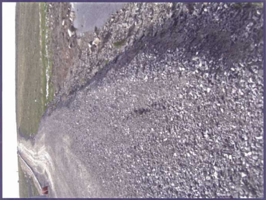
Photo 228 shows a longitudinal tension crack near the crest edge on the upstream side. This crack is related to the oversteepened slope immediately to the right.
