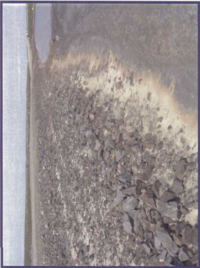
Photo 45 shows some sand which has blown off the crest and has accumulated at the toe of the upstream side against the tailings.
