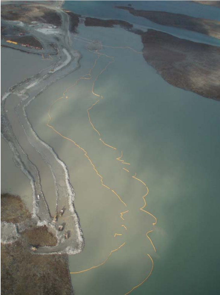
Photo 3-8. Compromised turbidity barriers on the east side of the Bay-Goose Dike work zone, 3 September 2009 (Day 38).
