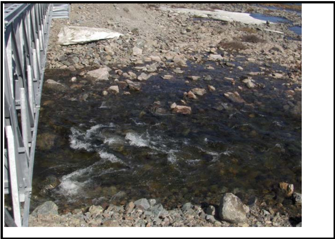
Photo No 9 : Immediately downstream of the bridge R02 - water levels subsided significantly (June 28, 2010).
