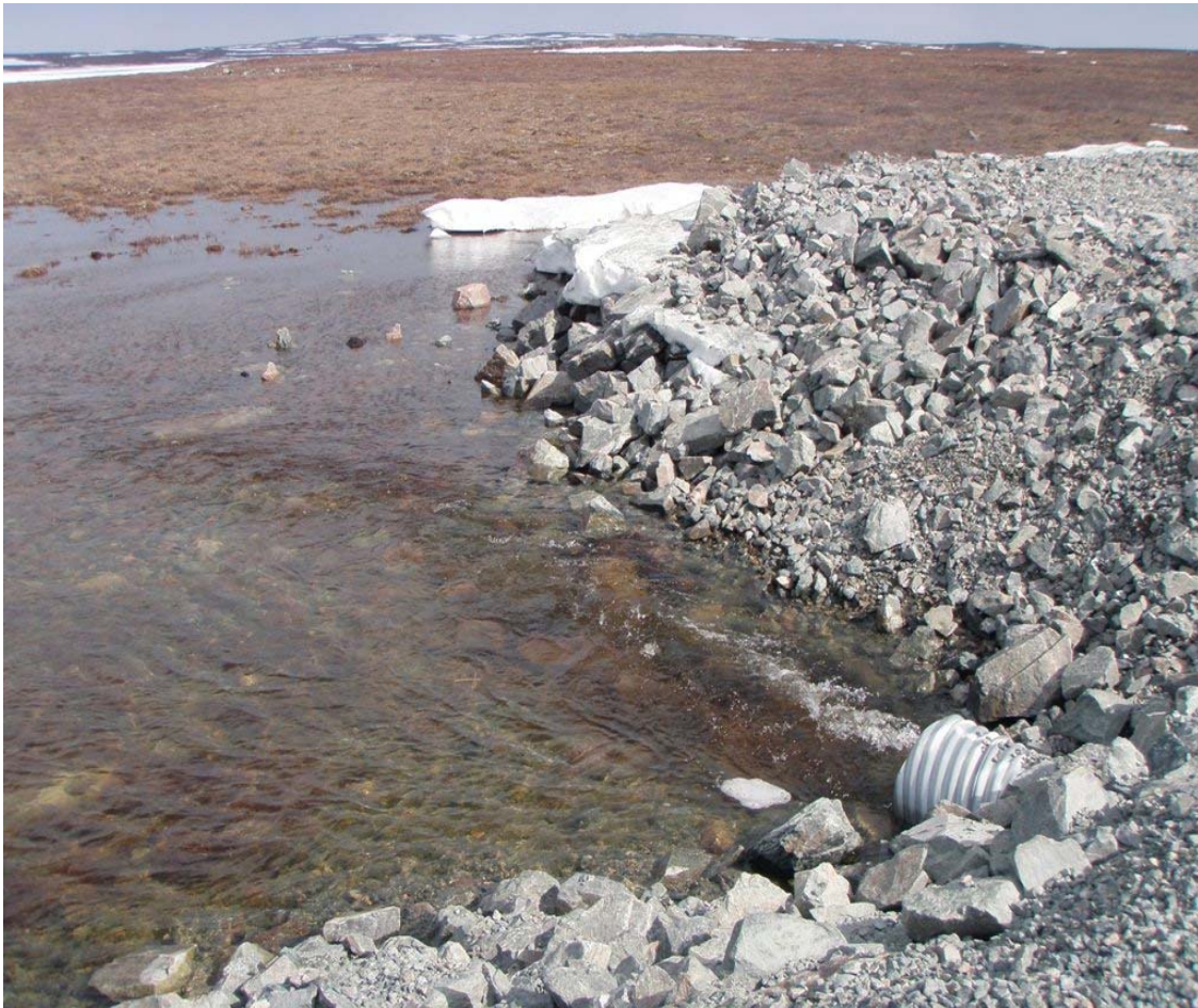
Standing Pool of Water draining to culvert at KM 20 – June 15, 2011
