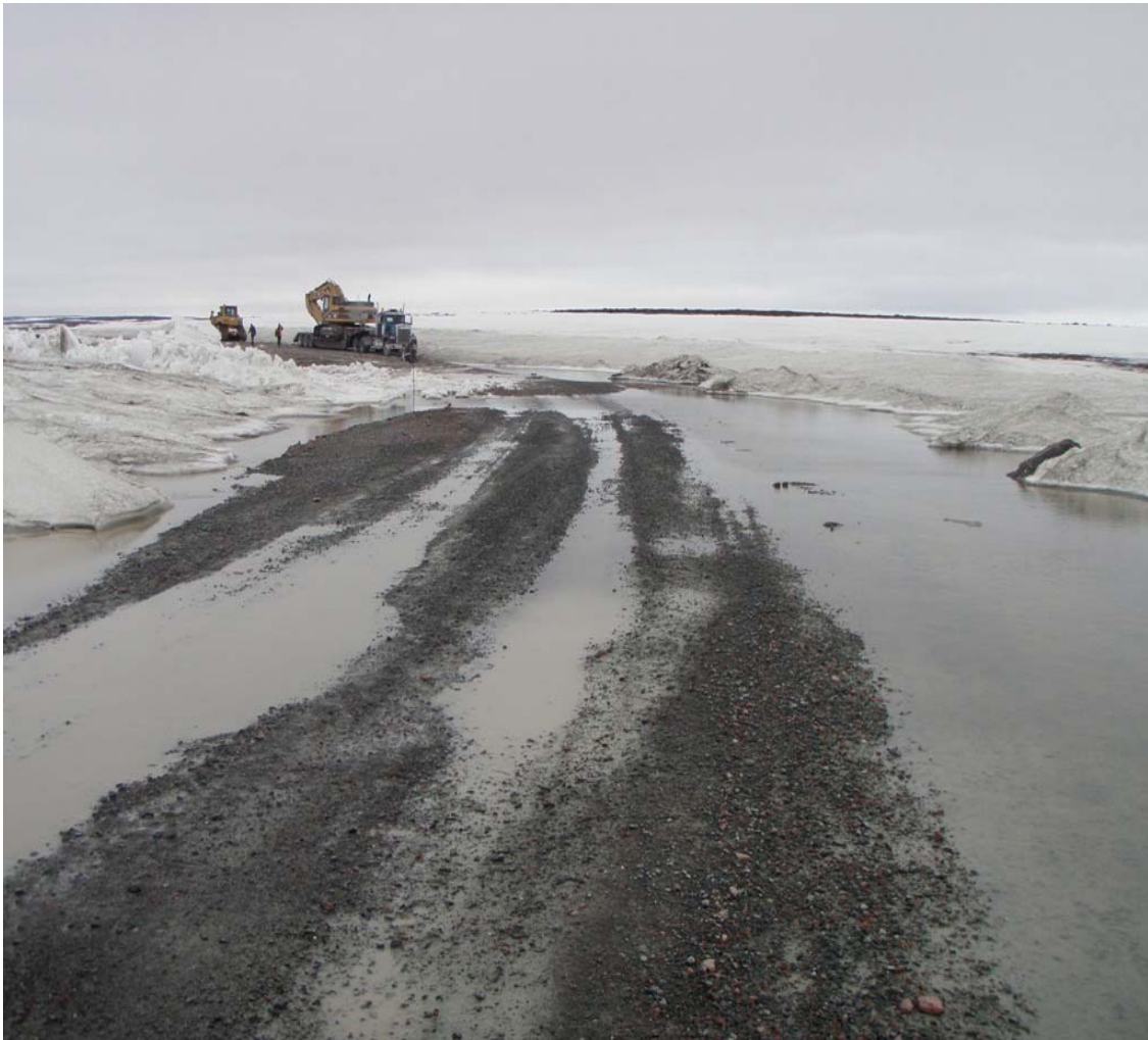
KM 80. Snow backing up culvert, blocking flow – June 15, 2011
