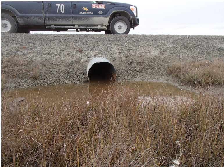
Photograph D1-27: unnamed km 13+950
