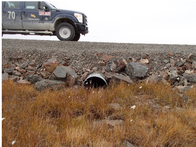
Photograph D1-17: R-03 km 10+580
