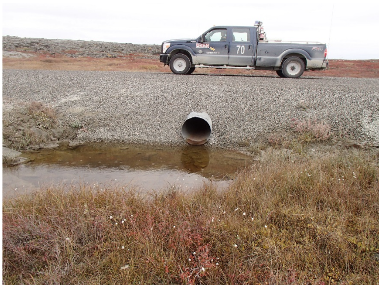
Photograph D1-28: unnamed km 13+950
