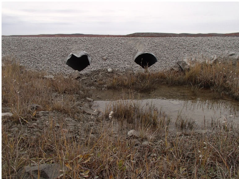
Photograph D1-37: PC-7A km 20+240
