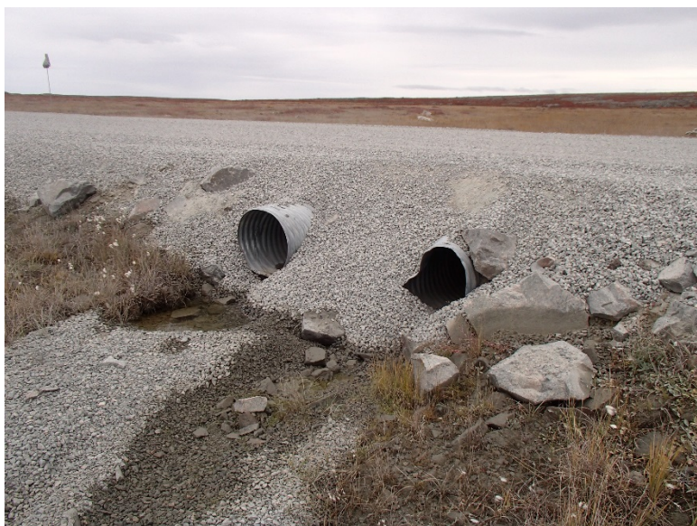
Photograph D1-38: PC-7A km 20+240
