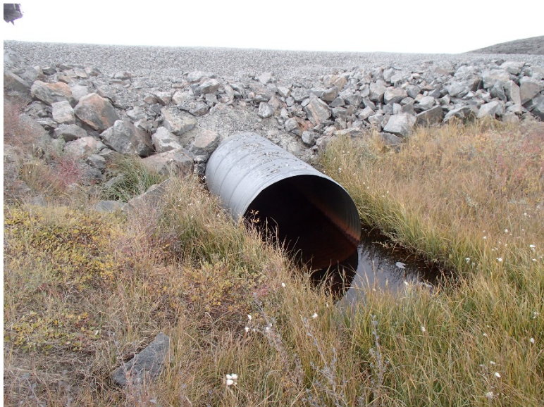
Photograph D1-31: R-05A km 15+745
