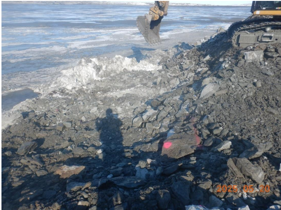
Exposure of natural ground for abutment tie-in and discovery of snow-rich material. Snow was removed prior to proceeding.
