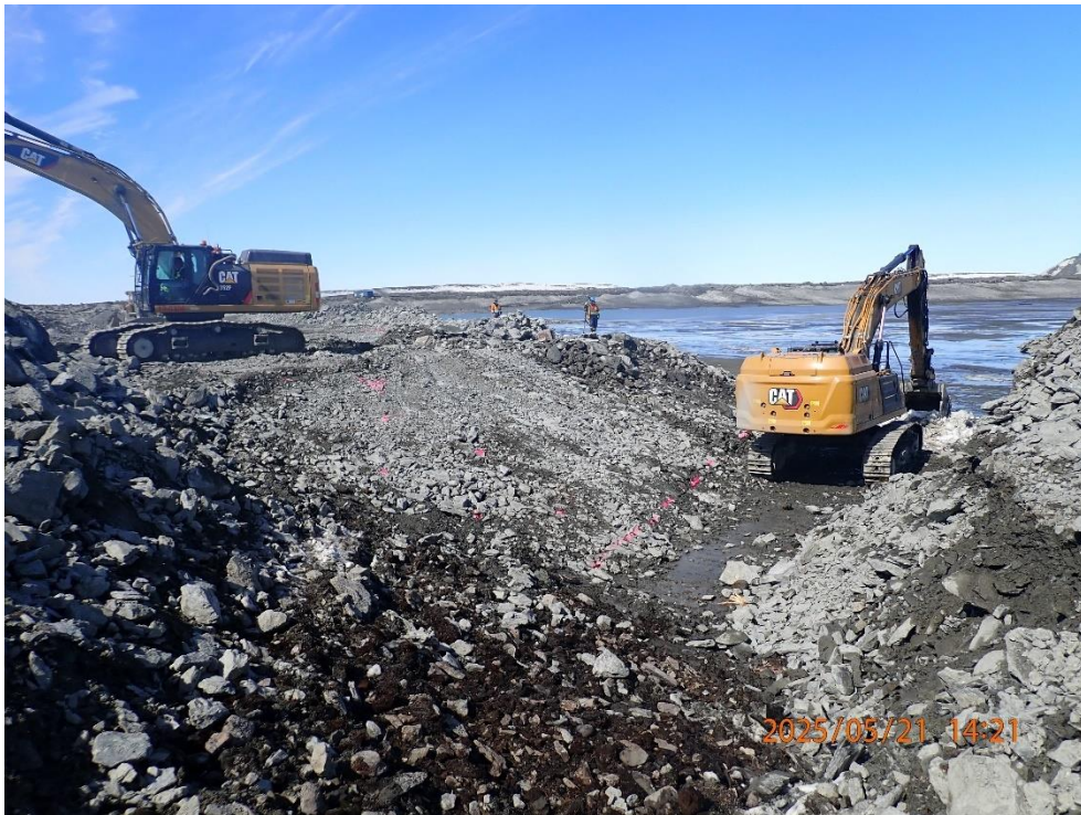
Sloping of rockfill material in preparation for geotextile placement at east abutment
