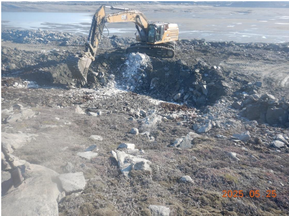
Non-compliant snow removal at west abutment
