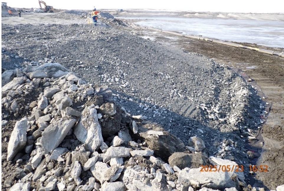
Completed placement and sloping of coarse filter near east abutment during road re-establishment to El. 145 masl
