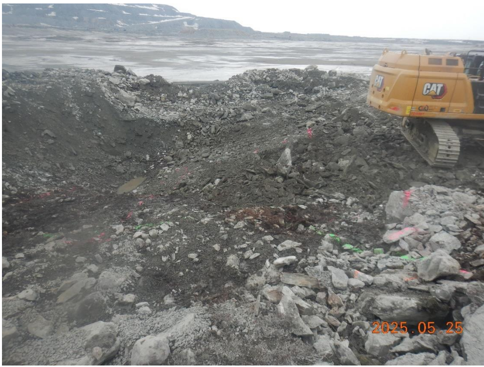
Exposure of natural ground at west abutment and slope preparation for geotextile
